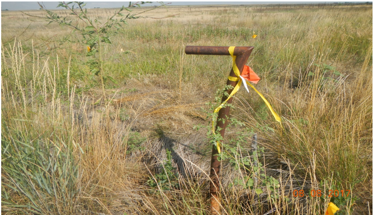
photo 2: The pipe riser identified in the previous inspection appears to be a vent pipe for pipeline.
