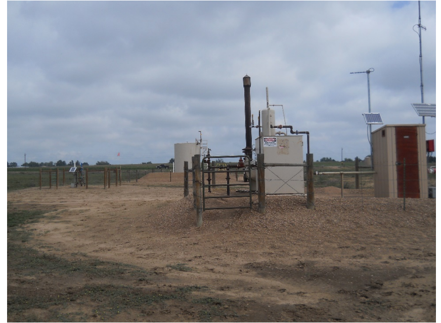
Battery looking north
