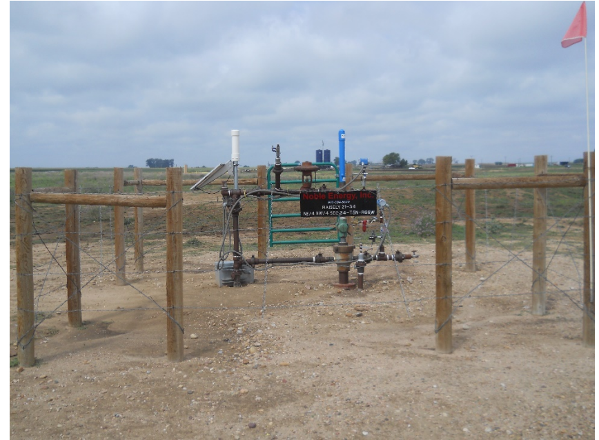
Wellhead looking west
