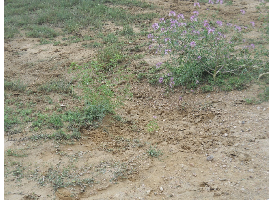
Location washing out northeast of tank battery (2/2 spots)
