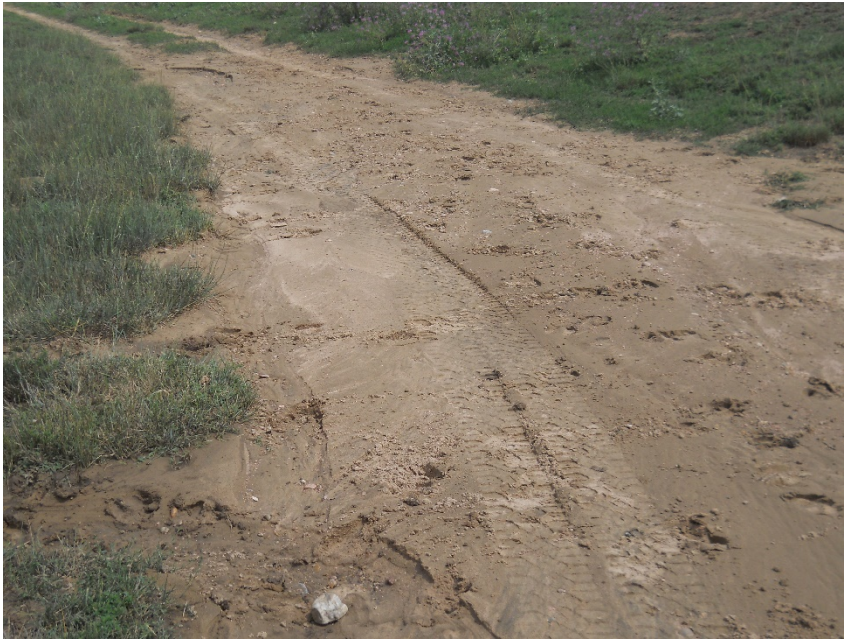
Lease road washing out headed northeast before curve
