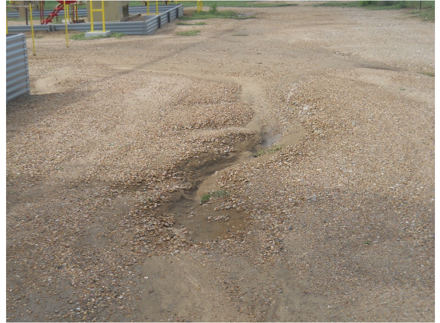
Another picture of location washing out west side of production tank
