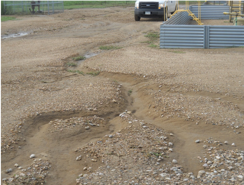
Location washing out northeast corner of tank berm
