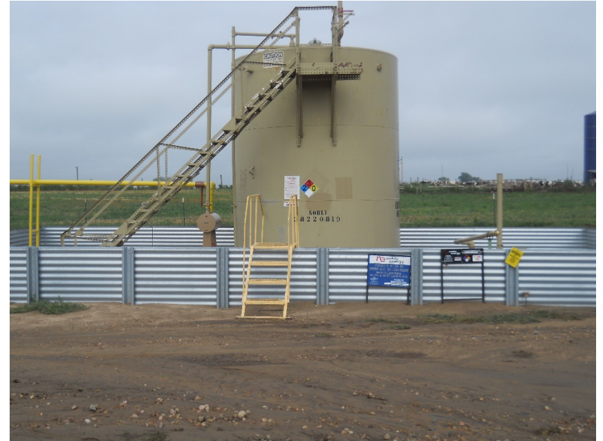
Tank battery looking west
