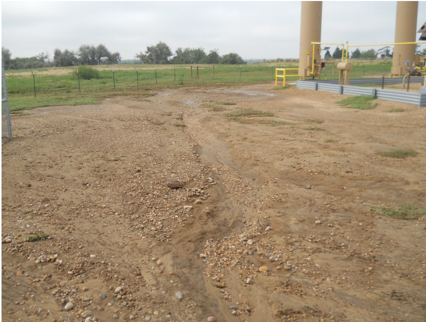
Location washing out southeast of tank battery
