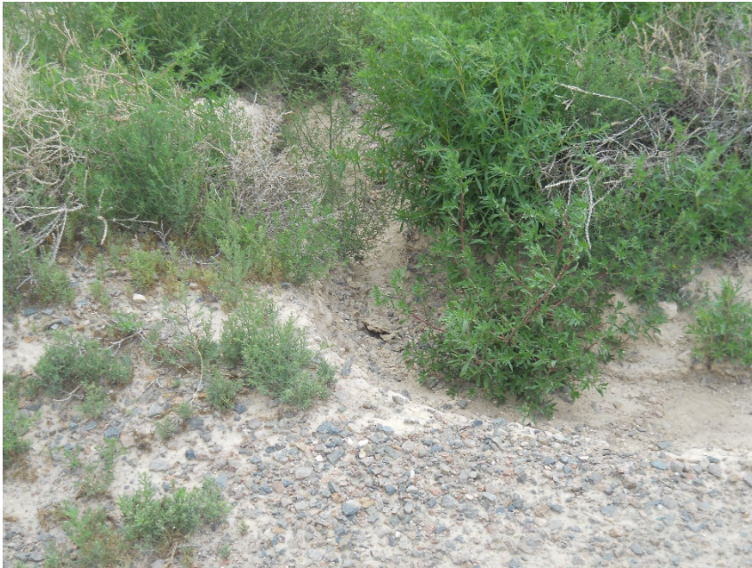
Erosion at entrance of location, west side
