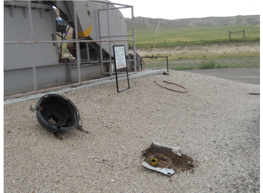
Trash on east side of pump jack
