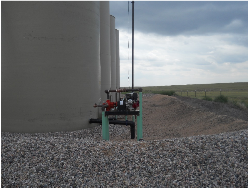
Production tanks looking south, recirc pump
