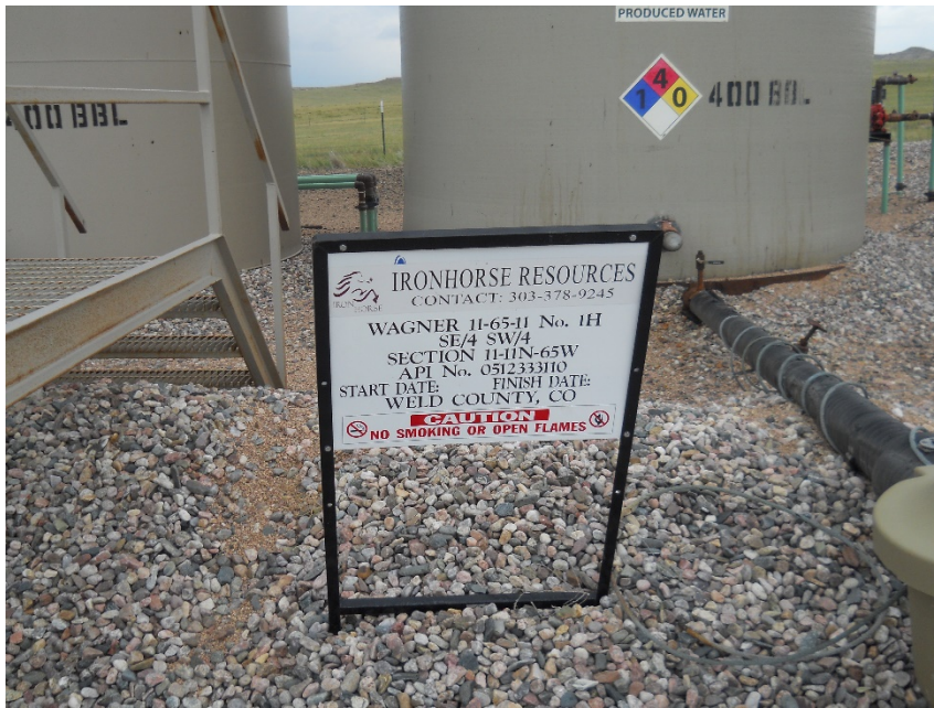
Battery sign east side of production tanks
