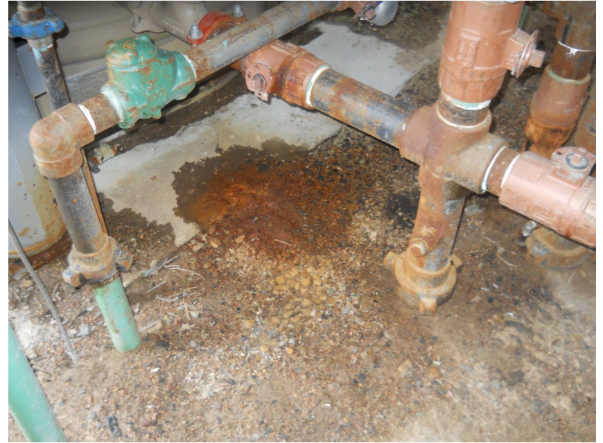
Stained soil inside of heater treater at oil and water inlets on south side
