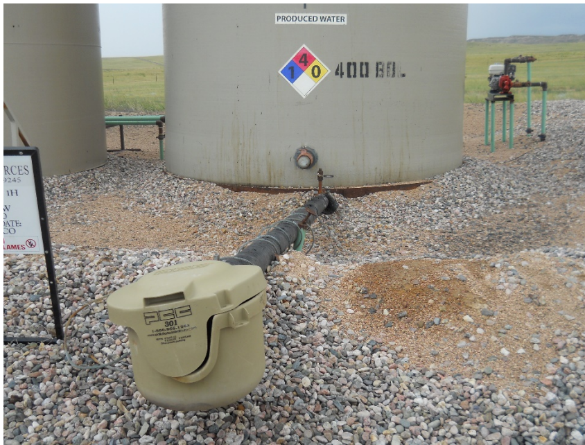
Unused 3" load line next to production water tank
