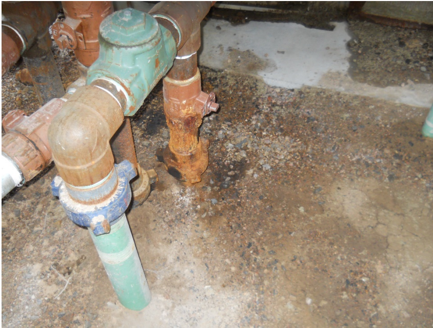
Stained soil inside of heater treater at oil and water inlets on the north side
