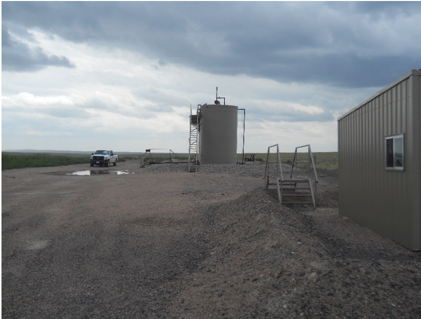
Battery looking south from heater treater
