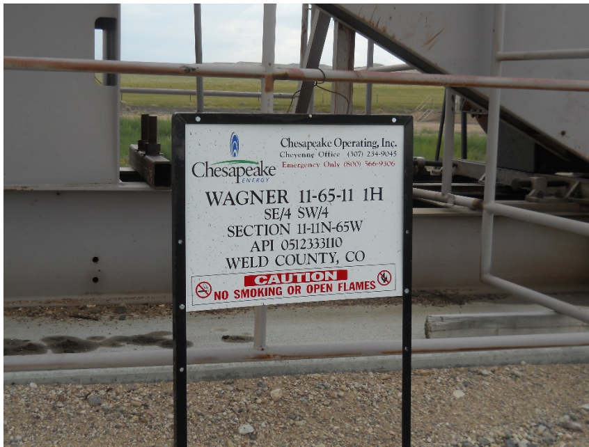
Wellhead sign with inaccurate operator information and inaccurate emergency contact information
