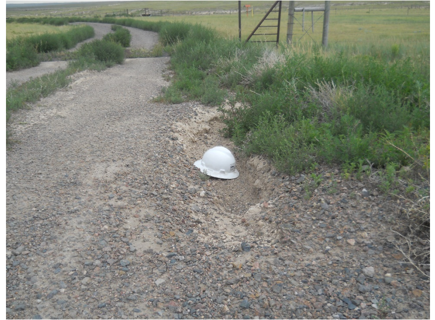
Erosion at entrance of location, west side
