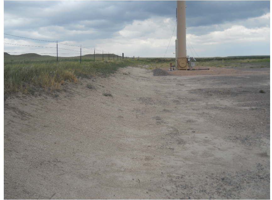
Sediment movement on cut slope at north end of location
