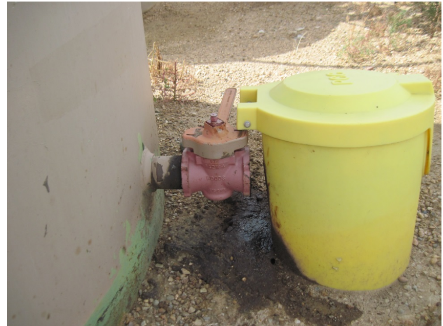
LOAD LINE VALVE NO CAP ON VALVE and stained soil
