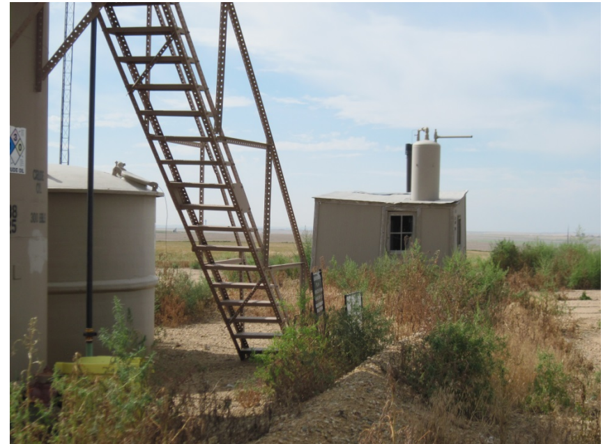
WEEDS AROUND BATTERY
