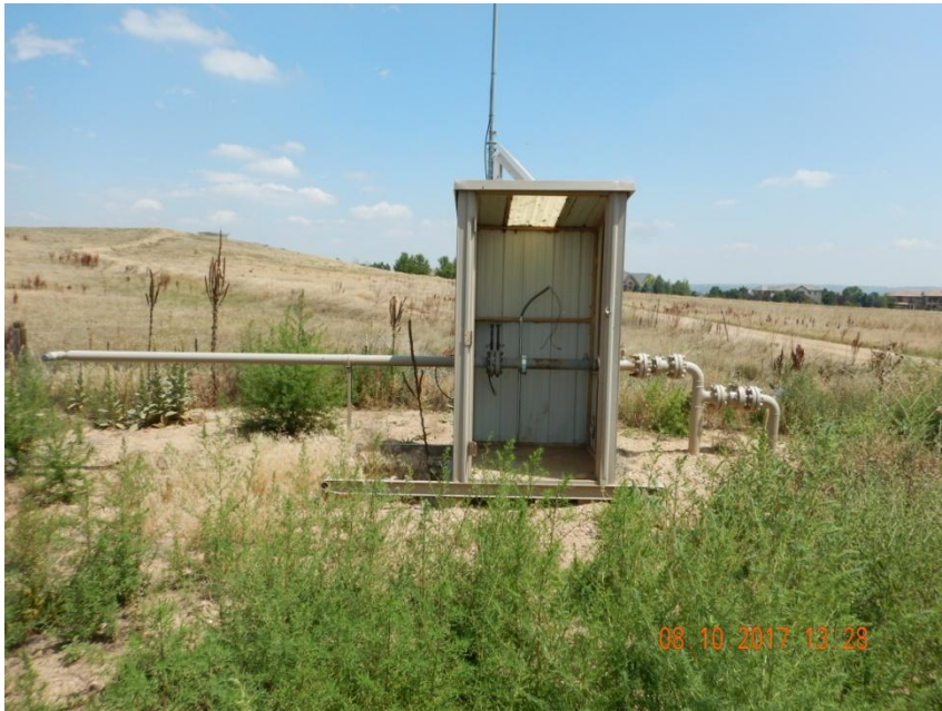
Photo 3. Photo taken of the meter shed observed along the eastern tank battery, facing East. As of August 10, 2017, the meter shed still remains at location.
