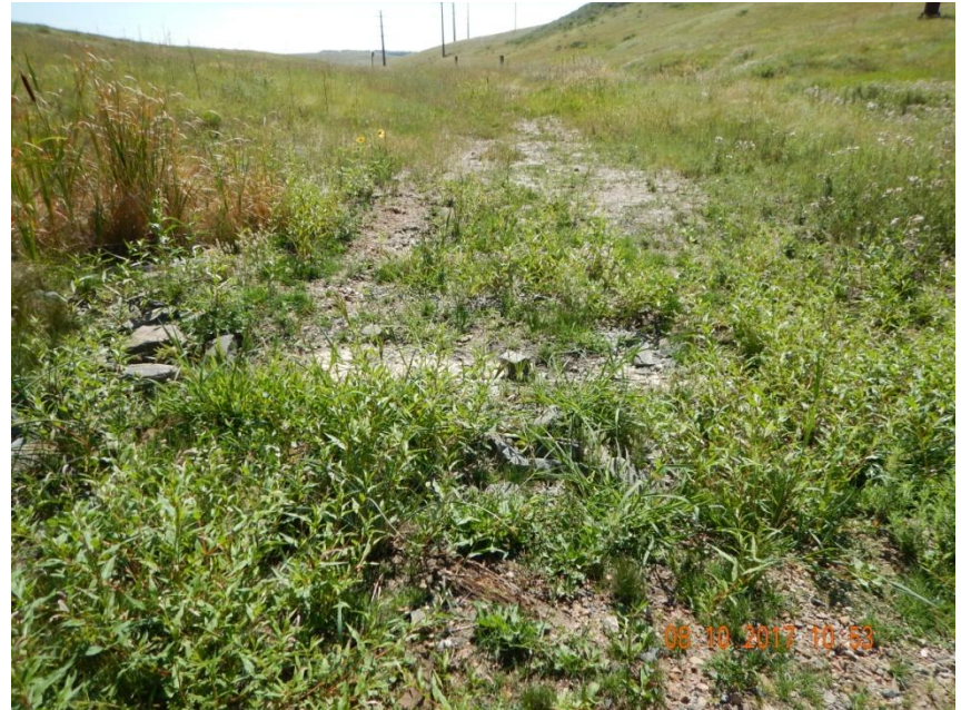
Photo 3. Photo taken from Culvert #1, facing East. Culvert has been removed and no stormwater erosion was observed.
