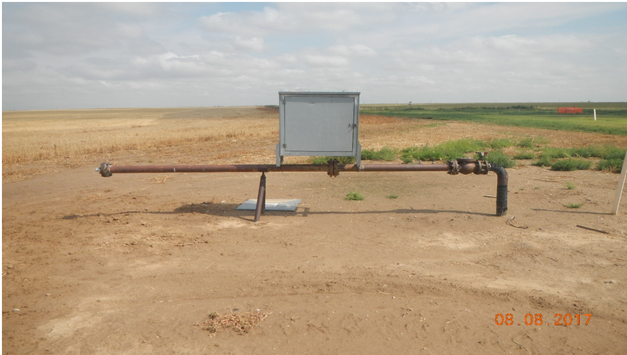
photo 4: There is an abandoned riser that remains at Lat/Long:39.84450,-104.45200.
