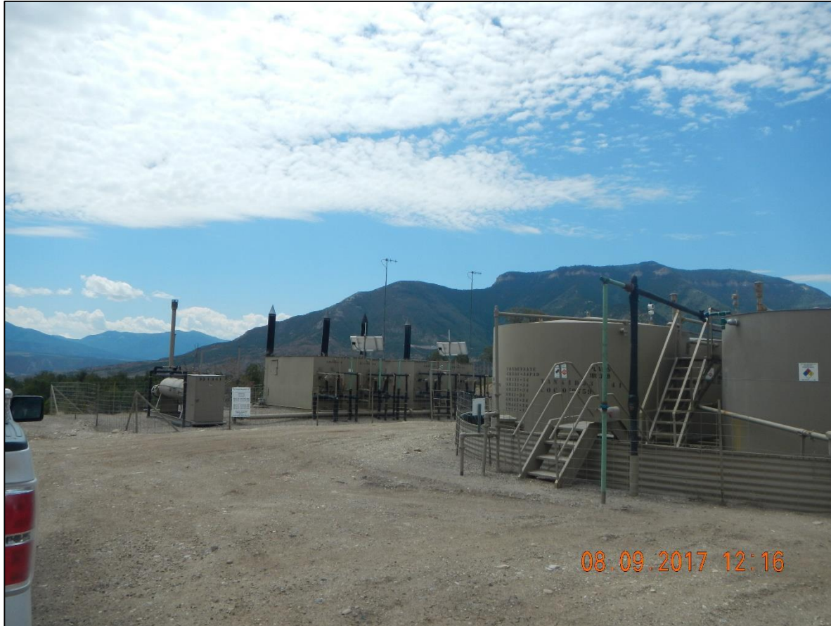
Separators and tank battery
