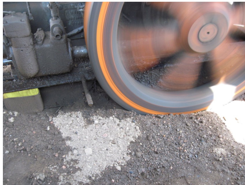
SOILD DIRT AROUND FLYWHEEL AND MOTOR MOUNTS
