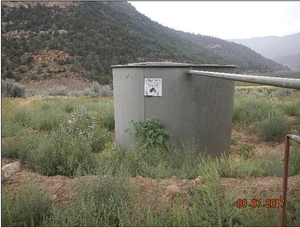
Photo 1. Weeds and vegetation in tank caontianment.
