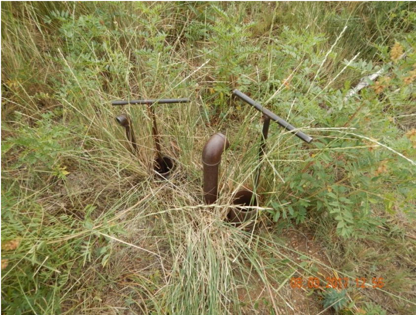
Photo 3. Close-up photo (1 of 2) taken of some of the pipe risers at location.
