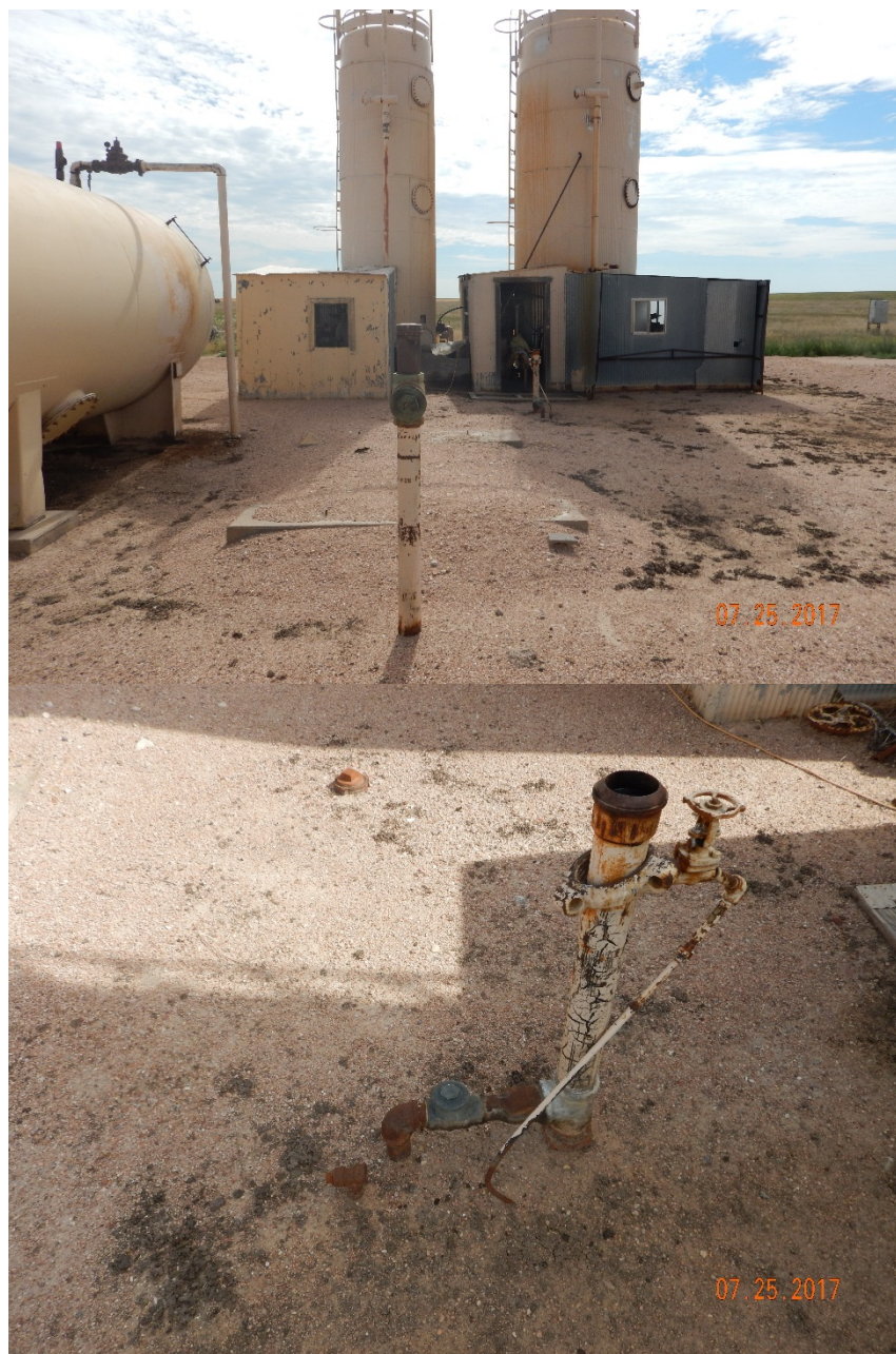
Figure 9 - Unused 4" flowline risers (top photo, foreground and background) located south of horizontal crude oil AST. Bottom photo shows 4" uncapped flowline riser, 1" riser, and 0.5" steel line just west of VHT sheds.
