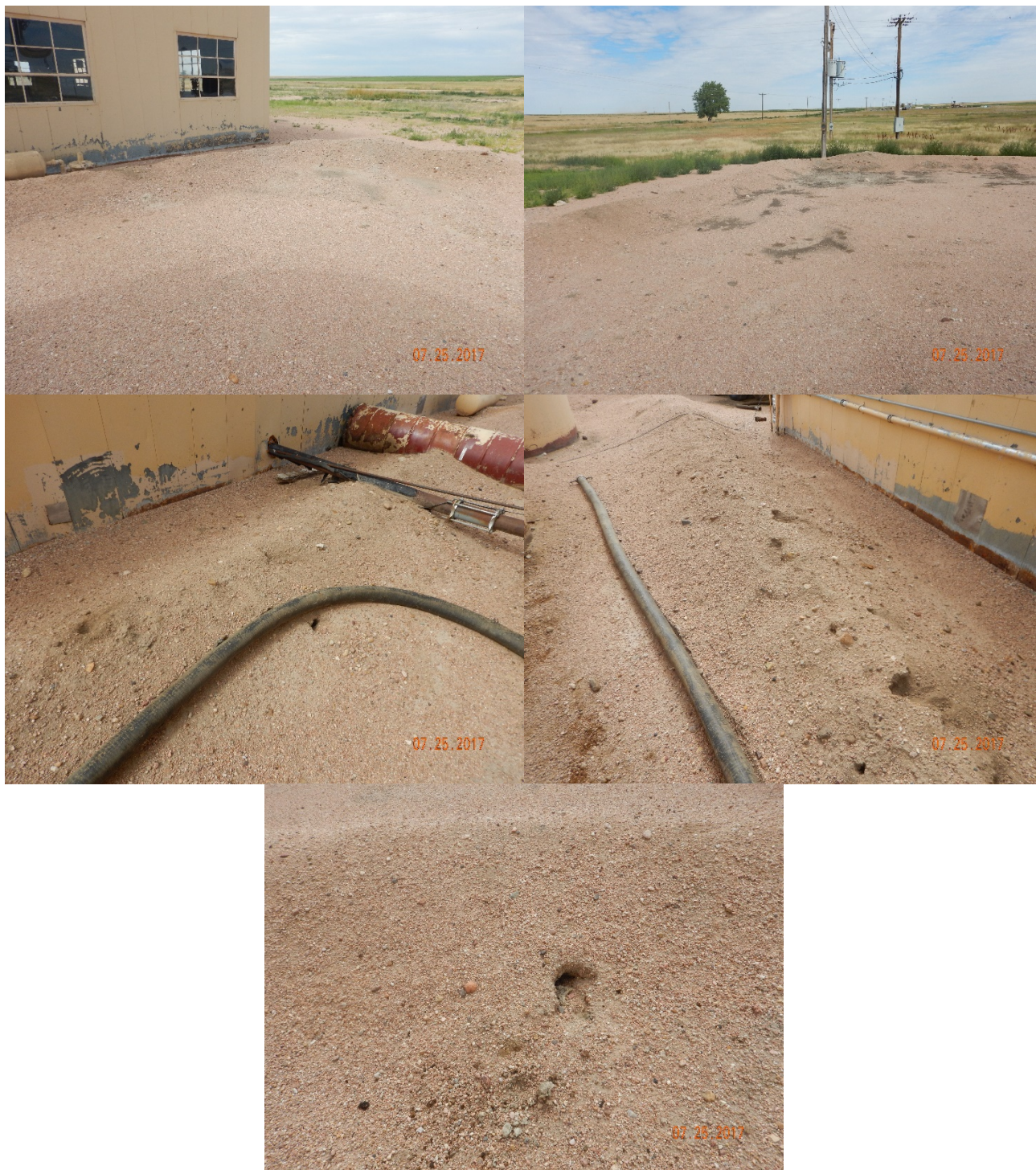
Figure 17 - Berm maintenance required for earthen berm around produced water ASTs.
