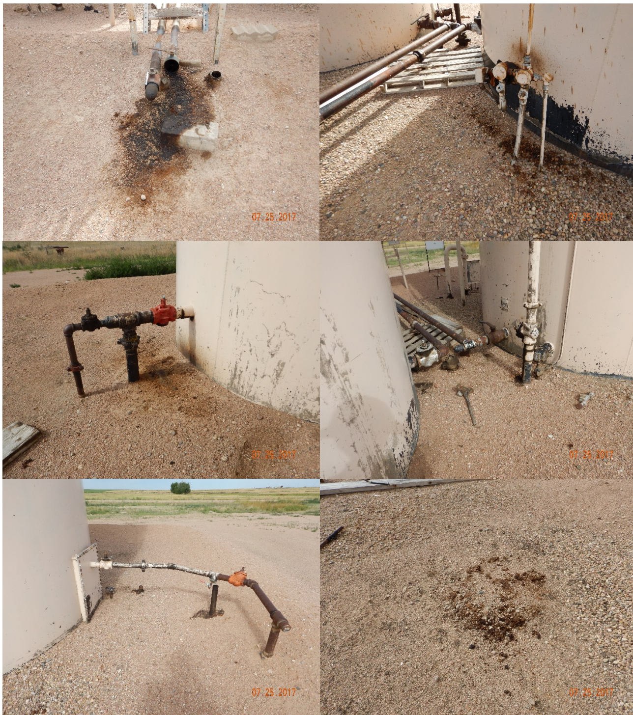
Figure 2 - Localized, oil-stained soil at multiple locations associated with crude oil ASTs.
