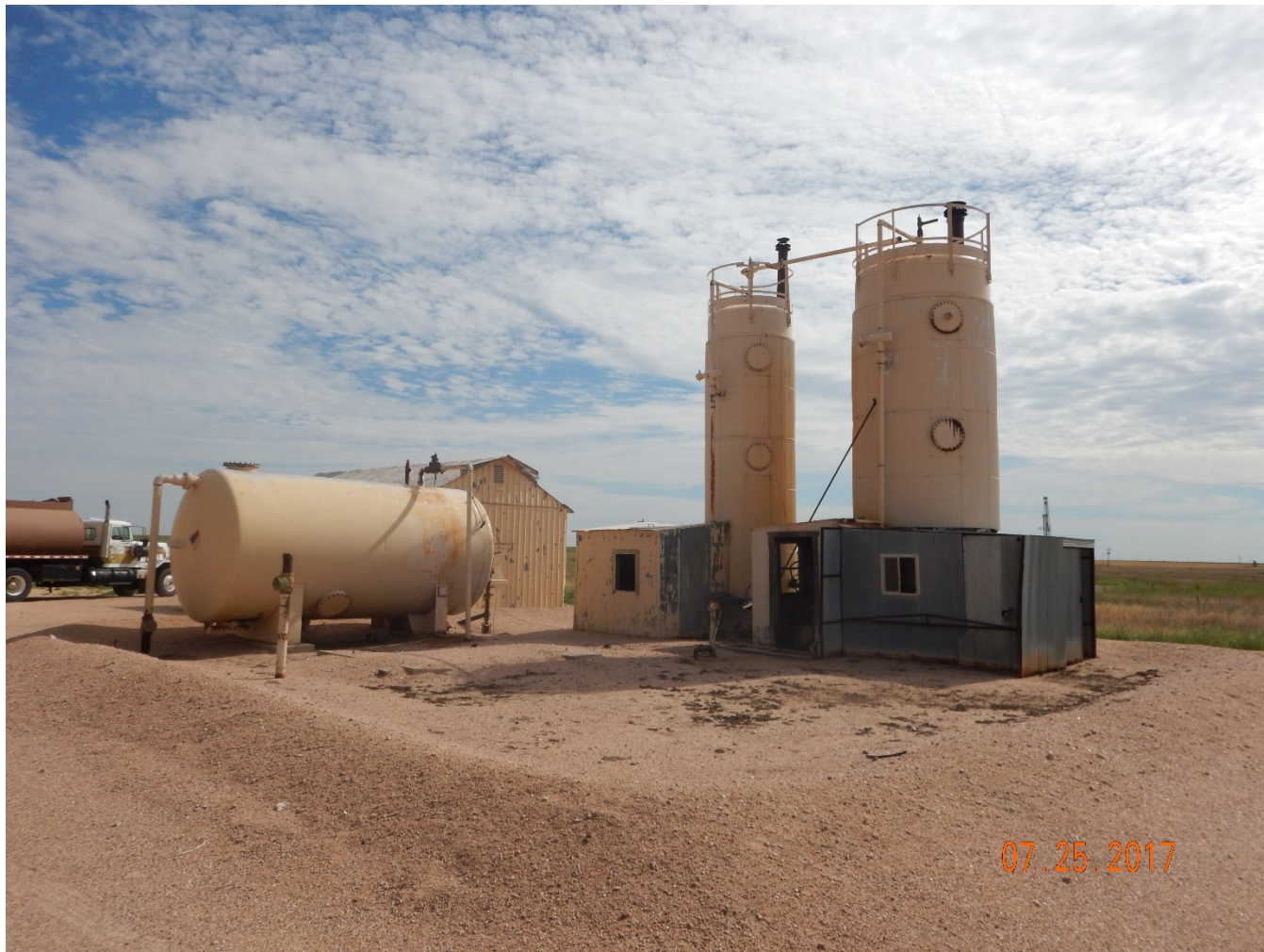
Figure 7 - Unlabeled horizontal AST and VHT sheds at SE corner of facility.
