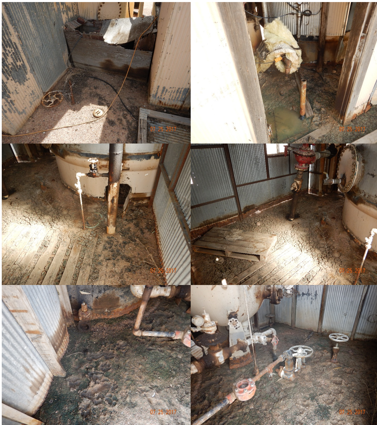
Figure 12 - Historical accumulations of oily waste, junk, and debris inside of VHT sheds.
