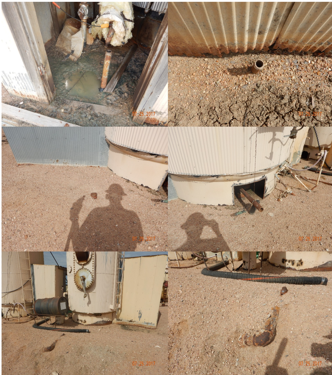
Figure 11 - Assorted flowline risers, pipes, and hoses (capped and uncapped) associated with VHT sheds.
