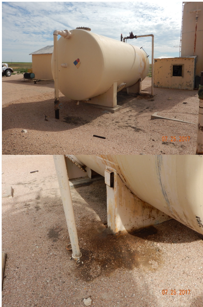
Figure 8 - Horizontal AST lacks volume and contents labels, NFPA placard needs replacement. Bottom photo: localized, oil-stained soil at SE corner of tank.
