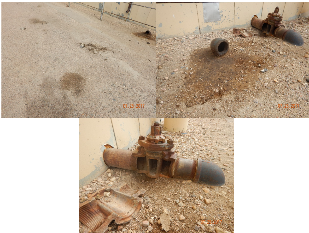
Figure 25 - Oily waste and irreparable flowline valve south of main injection building.
