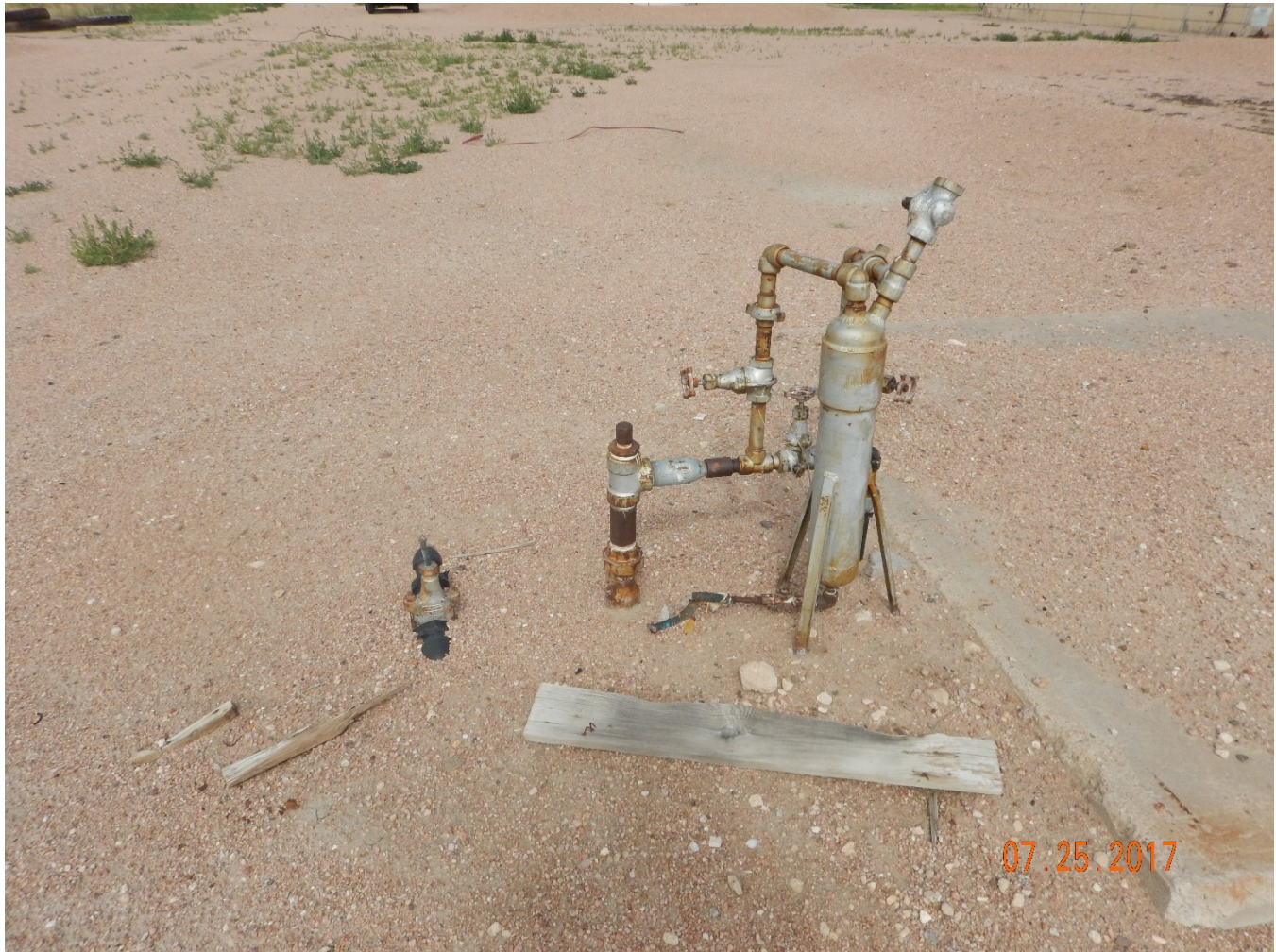
Figure 10 - Flowline manifold, wood debris, and concrete pad south of VHT sheds (outside of berm).
