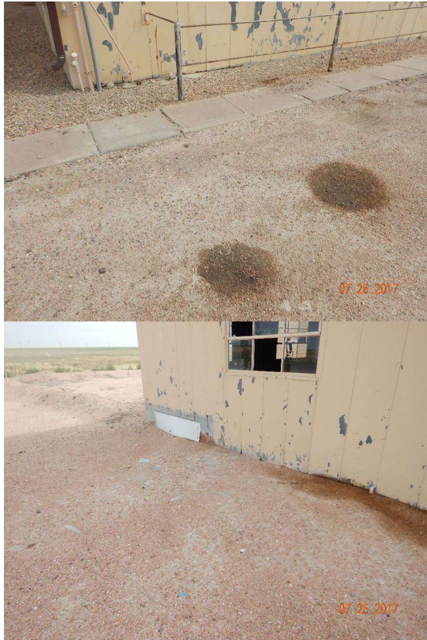
Figure 26 - Localized oily waste impacts at SW corner of main building (top photo) and with broken glass along west side of building (bottom photo).
