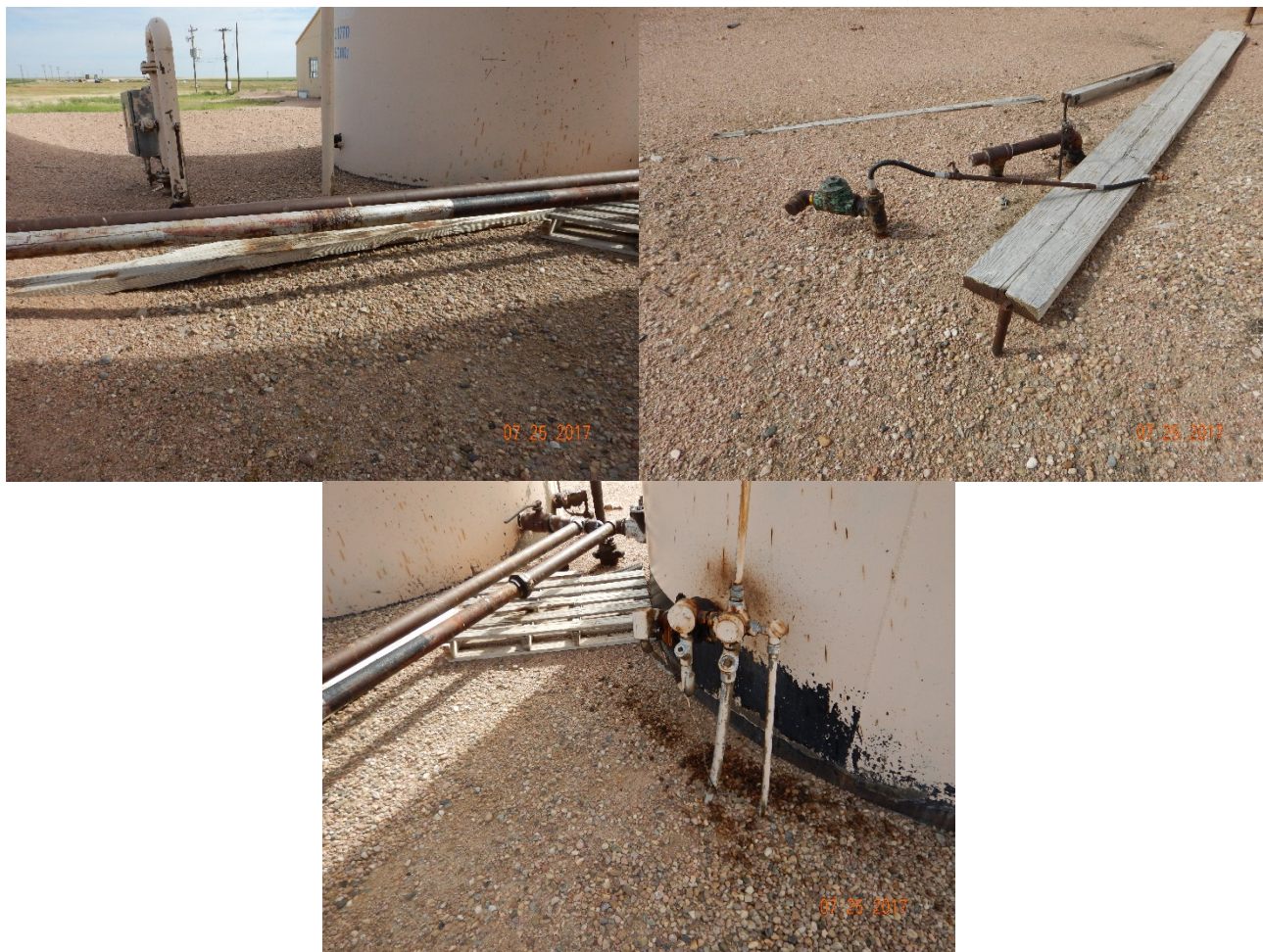
Figure 3 - Wood debris at crude oil ASTs.
