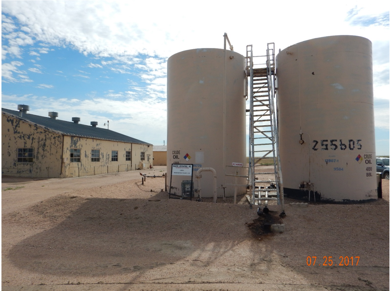
Figure 1 – Crude oil tanks at LBDSU Battery, COGCC Facility ID #451504. Note crude oil stain at truck loadout.
