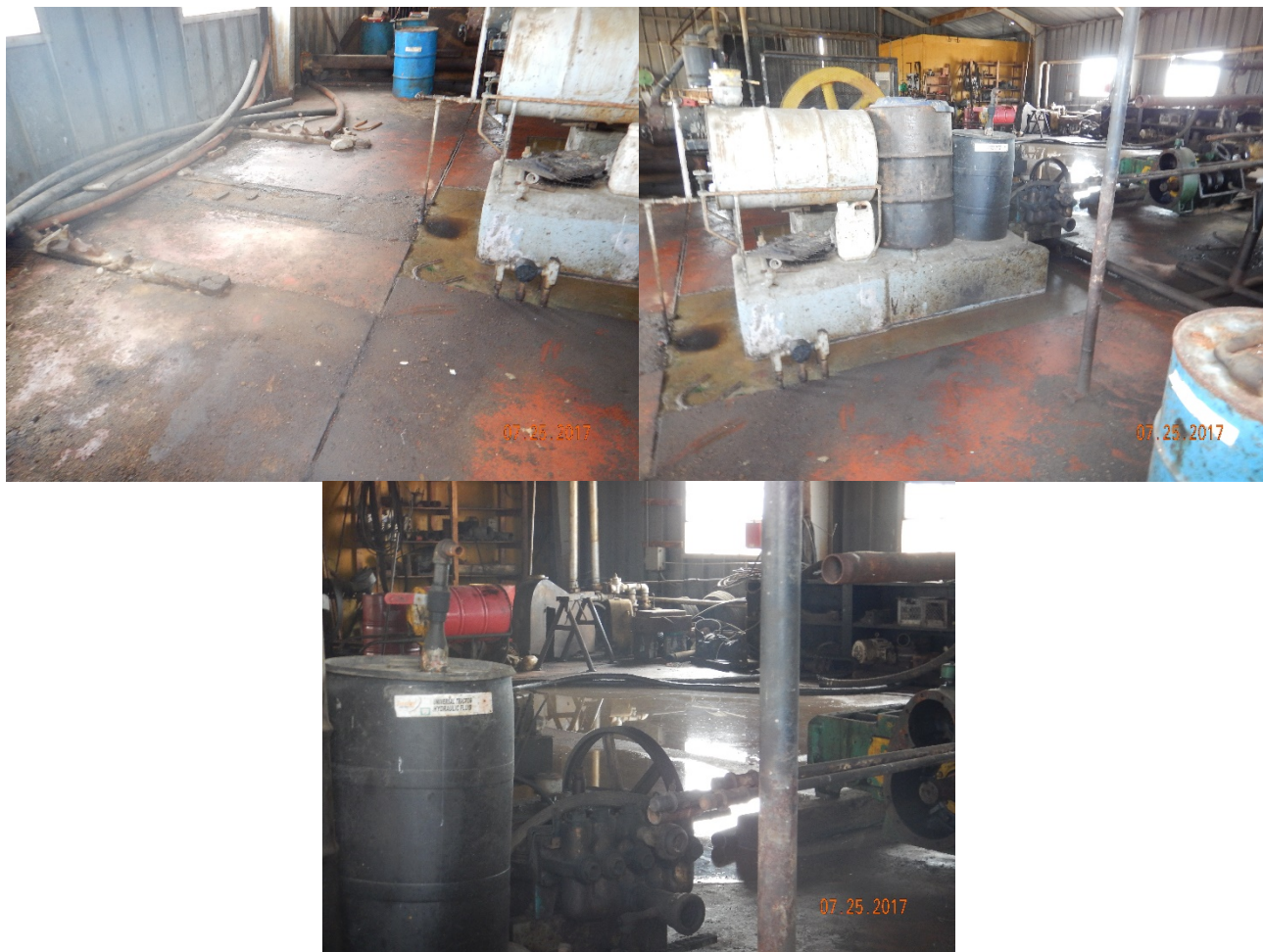
Figure 28 - Localized staining and large puddle in center of main building likely caused by leaking equipment.
