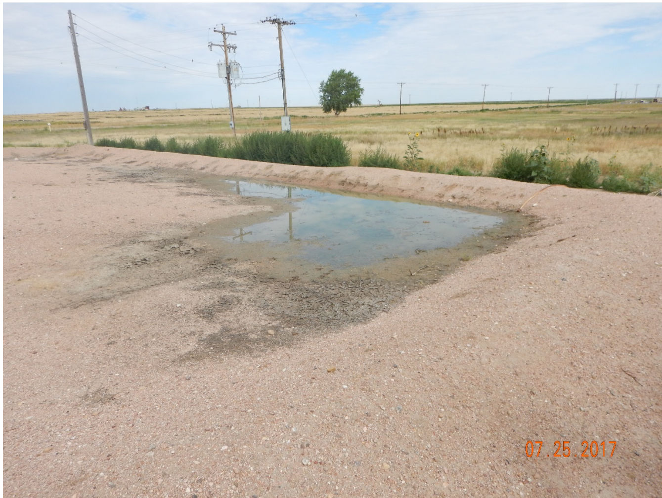
Figure 15 - Pool of water at NE corner of earthen berm around produced water tanks. Fluid source unknown.
