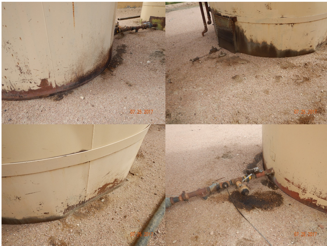
Figure 16 - Localized, oil-stained soil associated with produced water ASTs.
