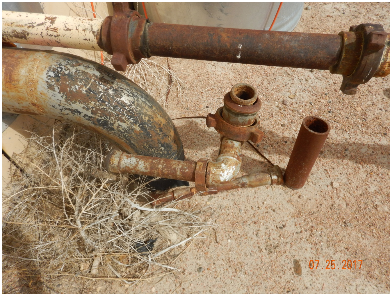
Figure 18 - Uncapped flowline risers at NE corner of injection plant.
