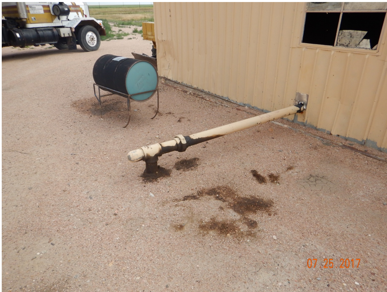
Figure 22 - Oily waste underlying flowline and 55-gallon drum south of vacuum truck.
