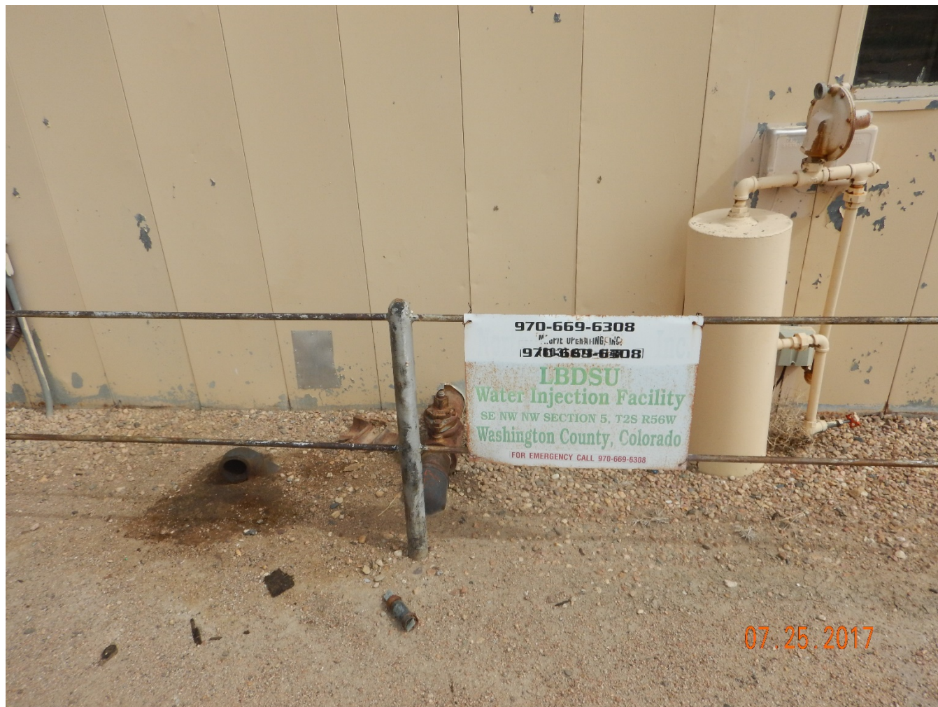
Figure 24 - Sign on south side of main injection plant, COGCC Facility ID #451505. Note; Localized, oil-stained soil at exposed pipes behind the sign.
