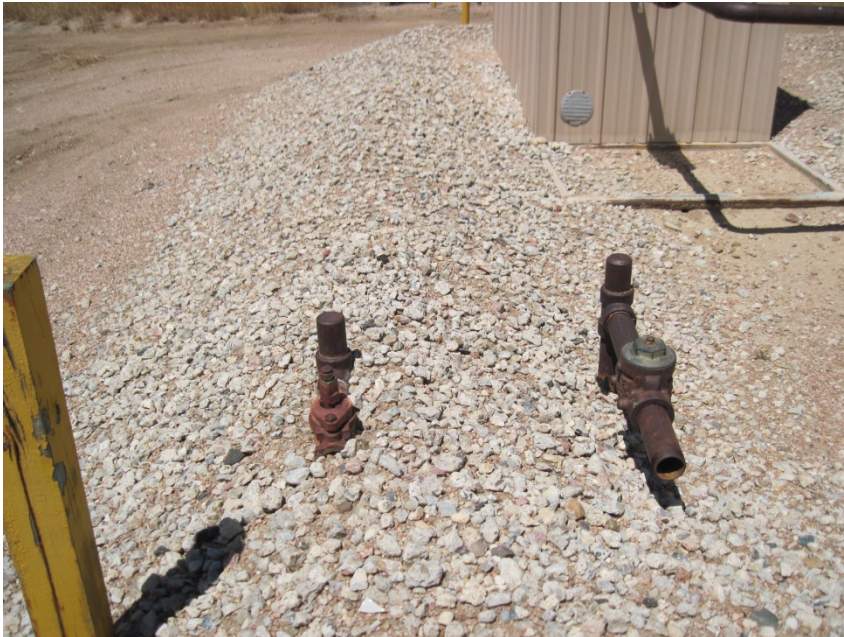
RISERS BT PRODUCTION UNIT
