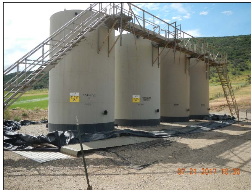
Photo 2. No berm around tank.
