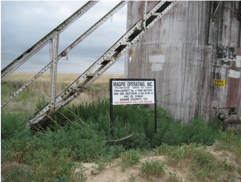
Tank battery, no capacity sign and weeds need maintained
