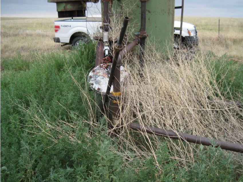
Unused equipment, scubber
