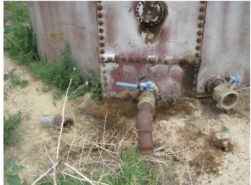
Staining on backside of tank
