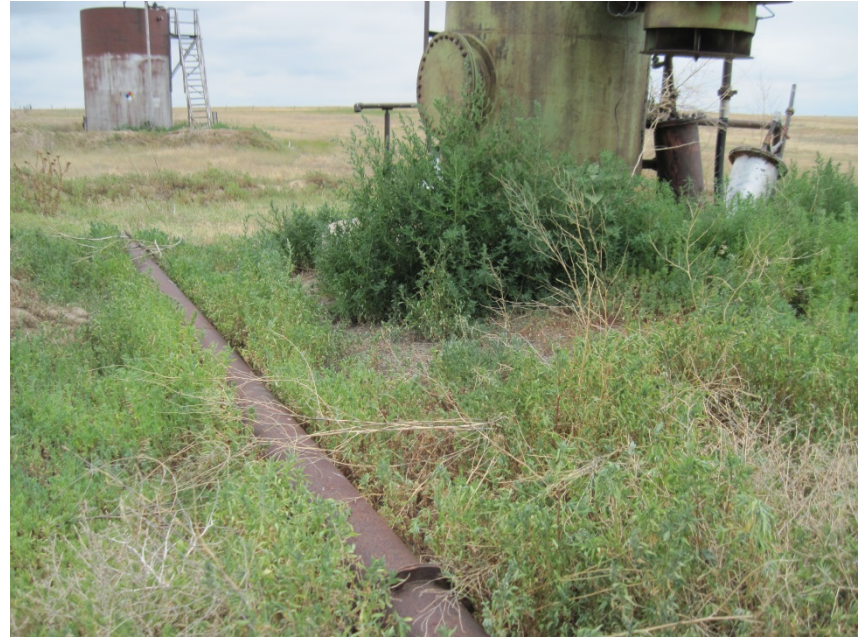
Unused equipment around treater
