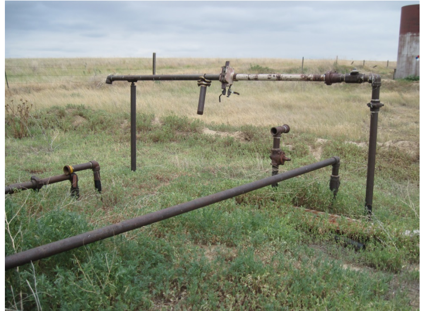
2 unmarked risers at meter run GPS N 39.90416 W - 103.77816
