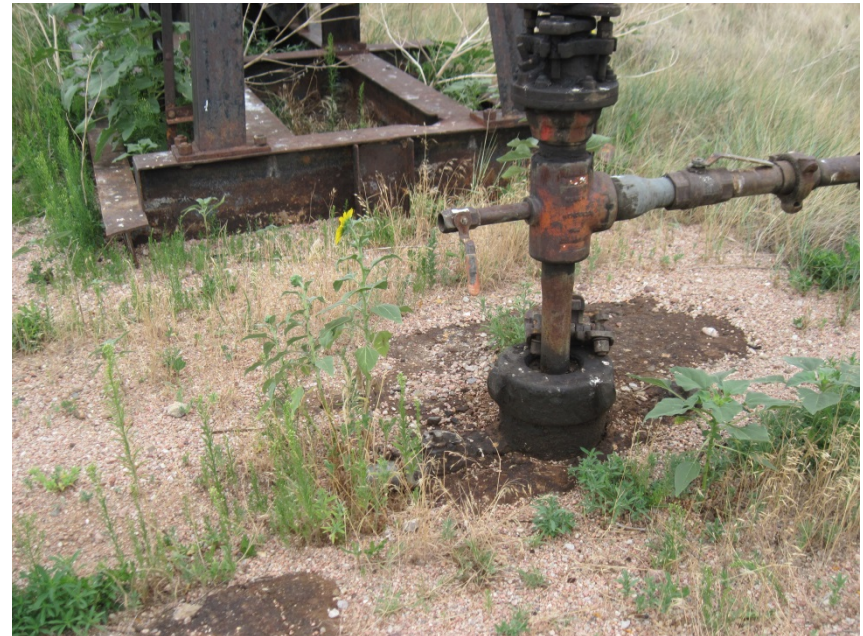
well location weeds on location, staining at wellhead
