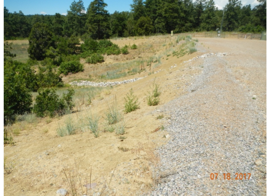
Photo 4: View of southern portion of the project area from the southeastern corner facing westward. Stormwater controls are in place.
