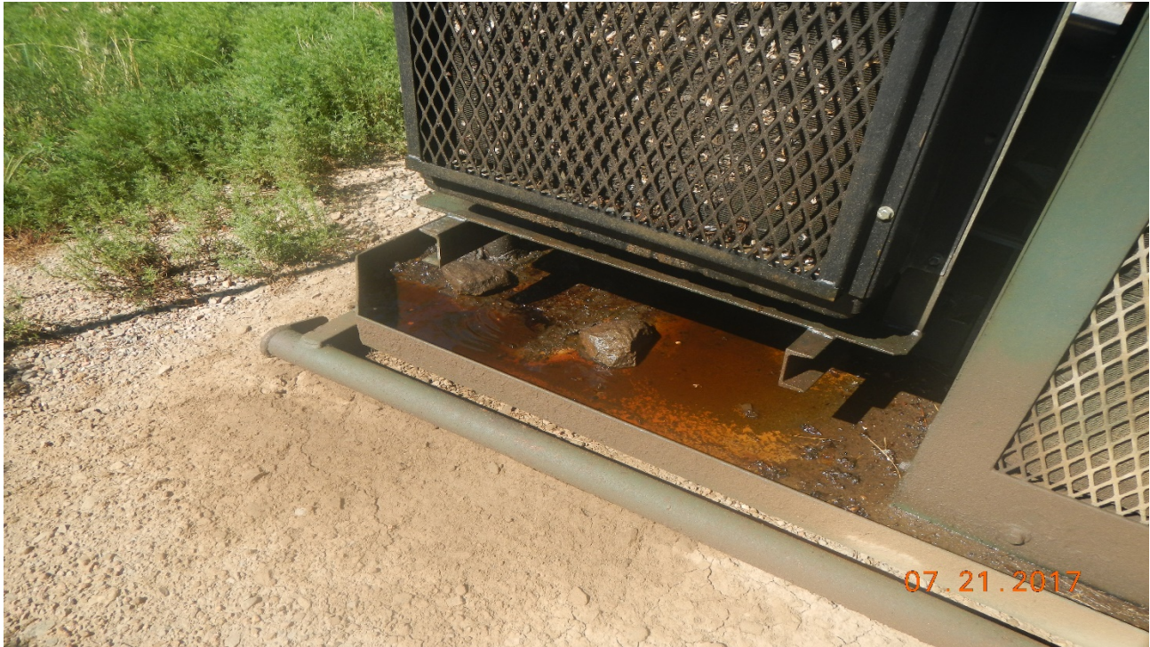
photo 5: There is oil on the engine skid.
