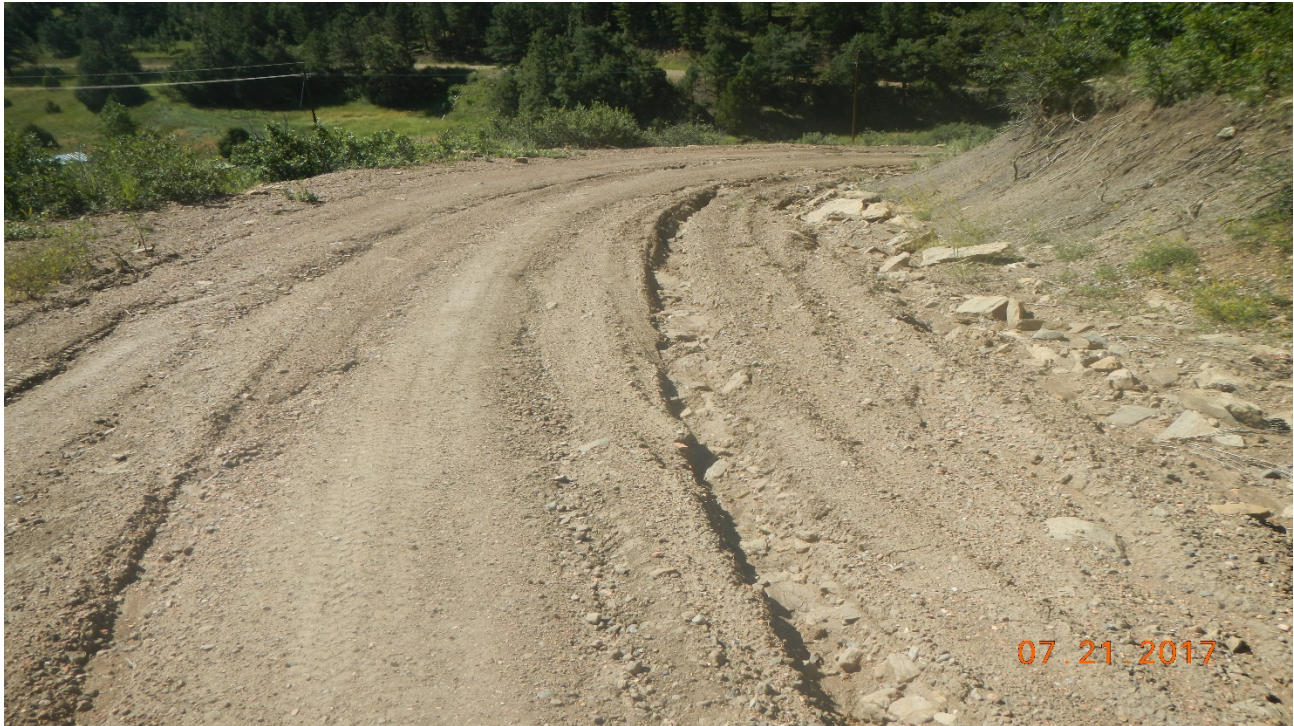
photo 3: Facing back along the main road. The ditches along the side of the road have filled in with sediment and stormwater is not properly diverted to the culverts.
