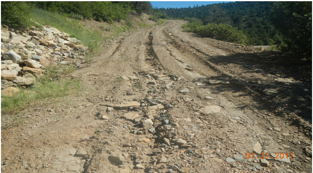
photo 2: Facing northeast along the main access road. Stormwater is not being properly diverted which is causing erosion along the road.
