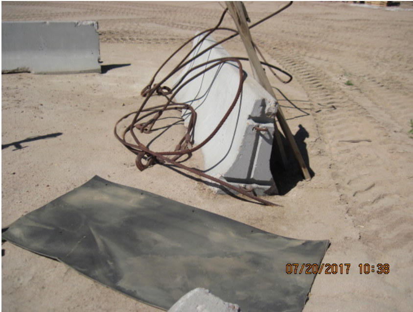
UNUSED EQUIPMENT BY WELLHEAD
