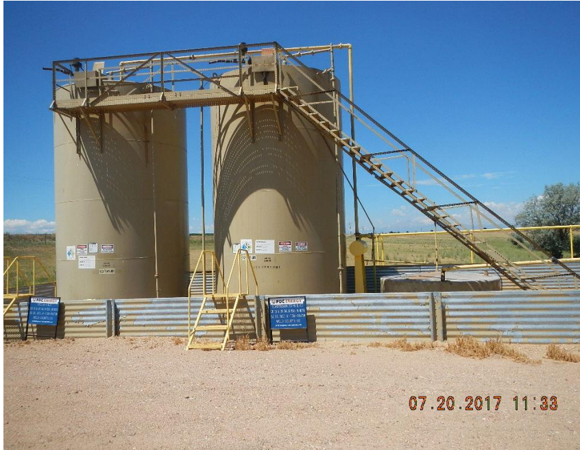
Photo 3 Tank battery from east
