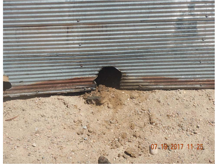
Photo 1: Stained soil at engine house
