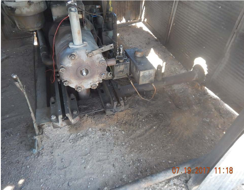
Photo 5: Stained soil in engine house
