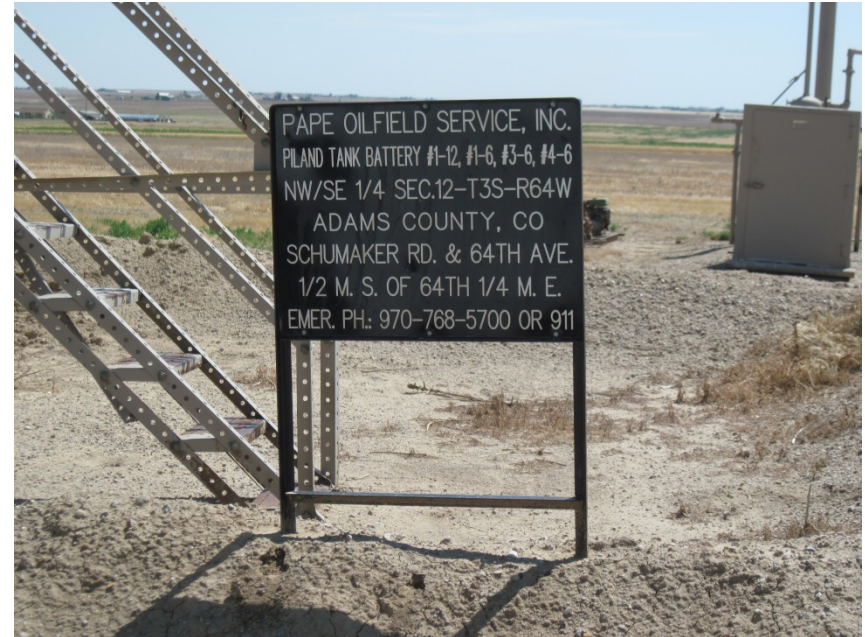
TANK BATTERY AND EQUIPMENT
