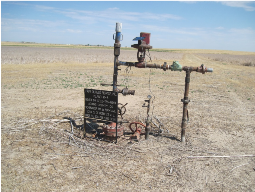
wellhead, intermitter controller
