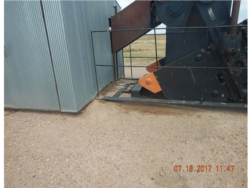
Photo 2: Stained soil at pump jack
