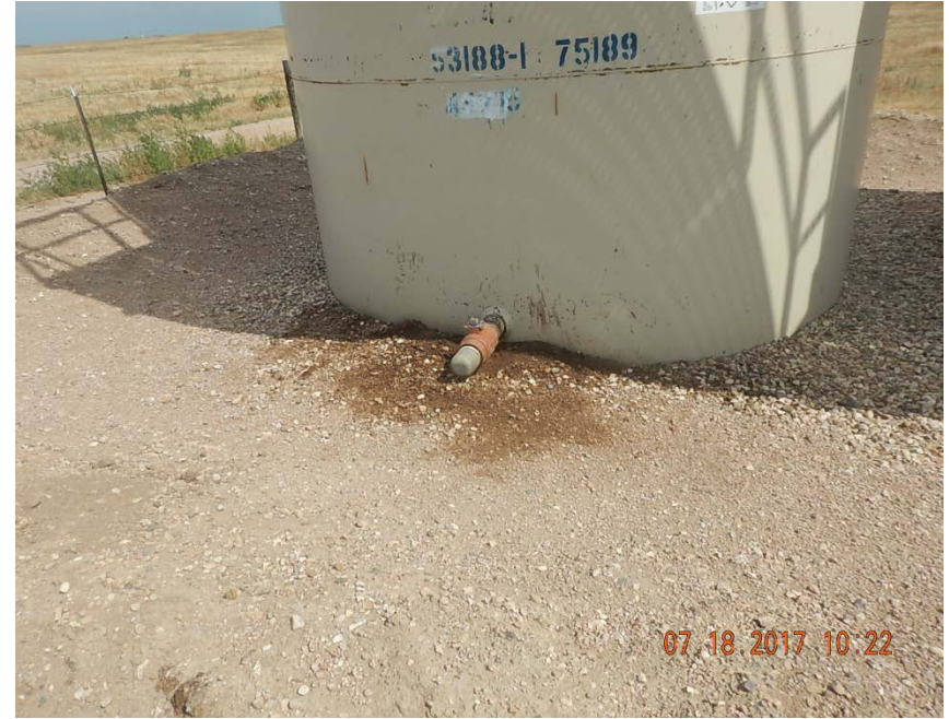
Photo 4: Stained soil at tank
