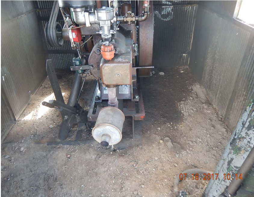
Photo 12: Stained soil at engine
