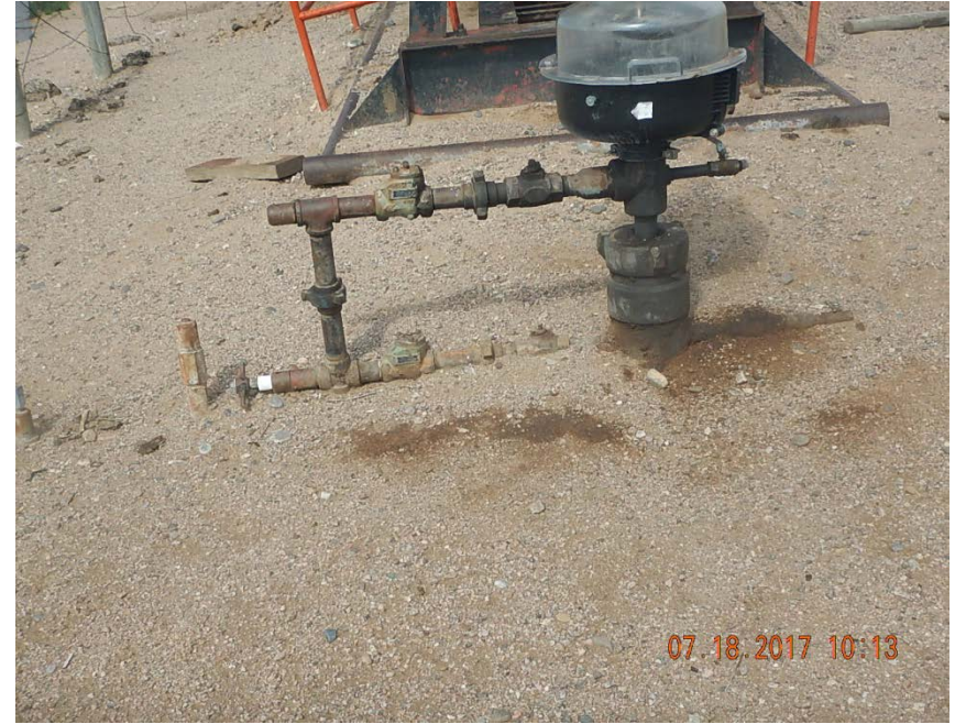
Photo 1: Stained soil at wellhead. One unused riser at wellhead.
