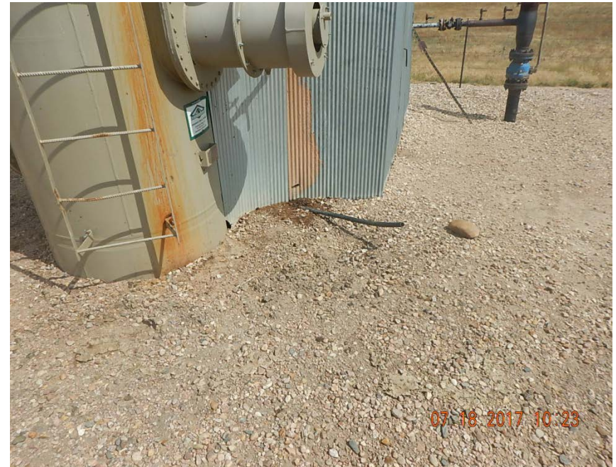
Photo 15: Stained soil at treater house
