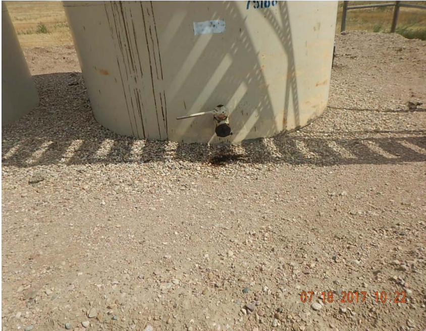
Photo 16: Stained soil at loadout valve
