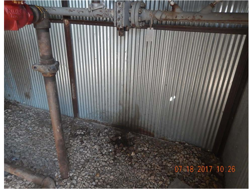
Photo 9: Stained soil in treater house
