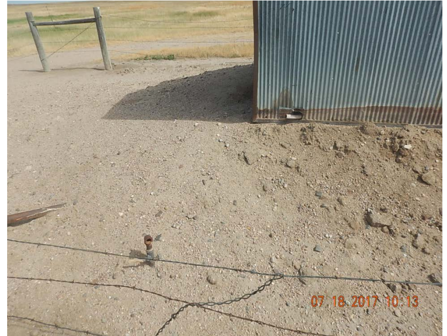
Photo 13: Unused riser at pump jack
