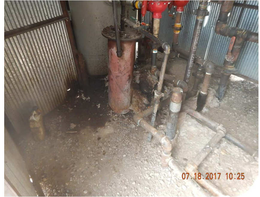
Photo 10: Stained soil in treater house
