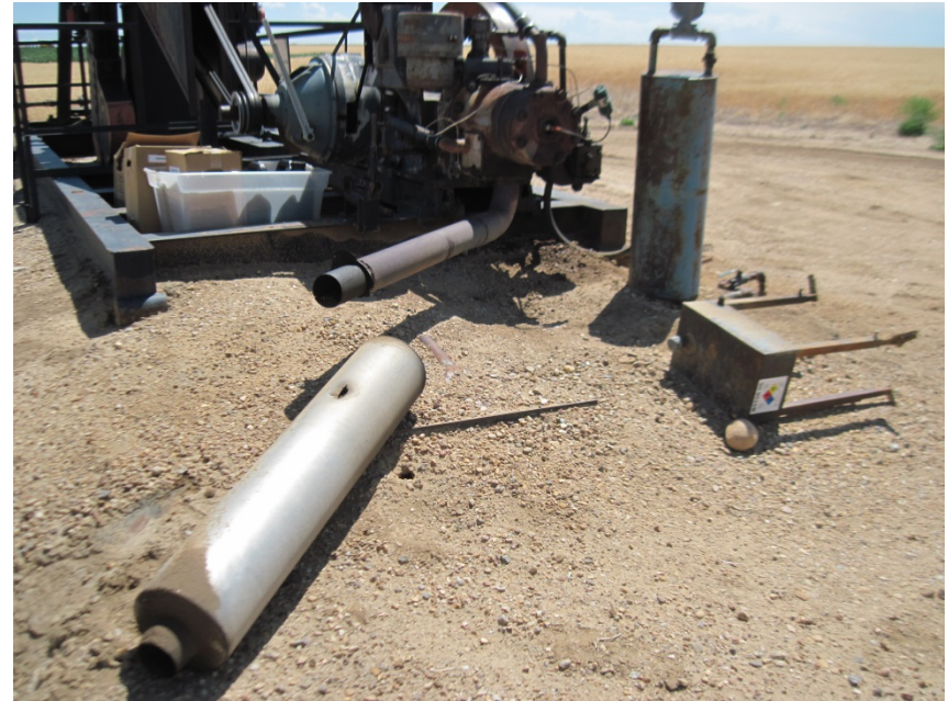
UNUSED EQUIPMENT AND SOILED DIRT
