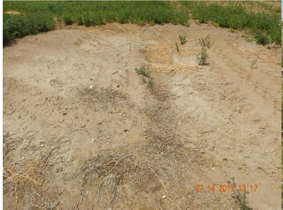
Photo 5: Photo taken from the well location. Photo shows subsidence occurring at well. Photo also shows that well does not appear to have been reseeded and area remains bare with no sign of germination or growth from the spring growing season.
