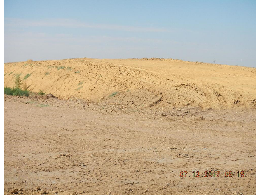
Photo 6 Top soil berm. NE corner GPS 40.18864, -140.67531 SW corner GPS 40.18750, -104.67548, approx. 15 ft thick
