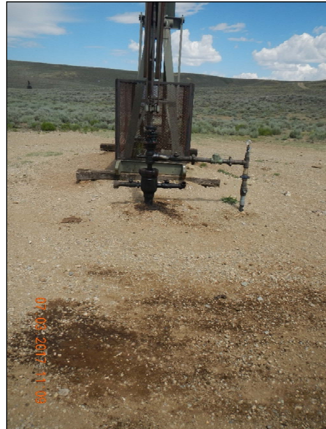
Photo 2. Stained soil at wellhead.
