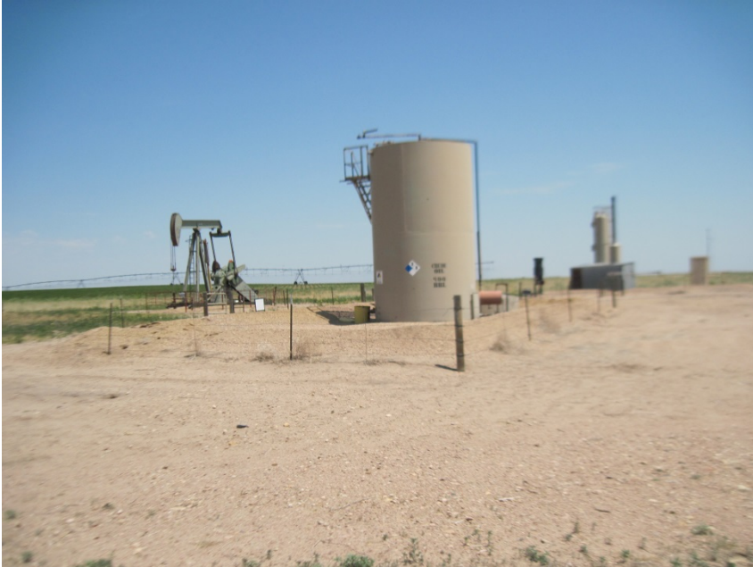
BATTERY AND EQUIPMENT
