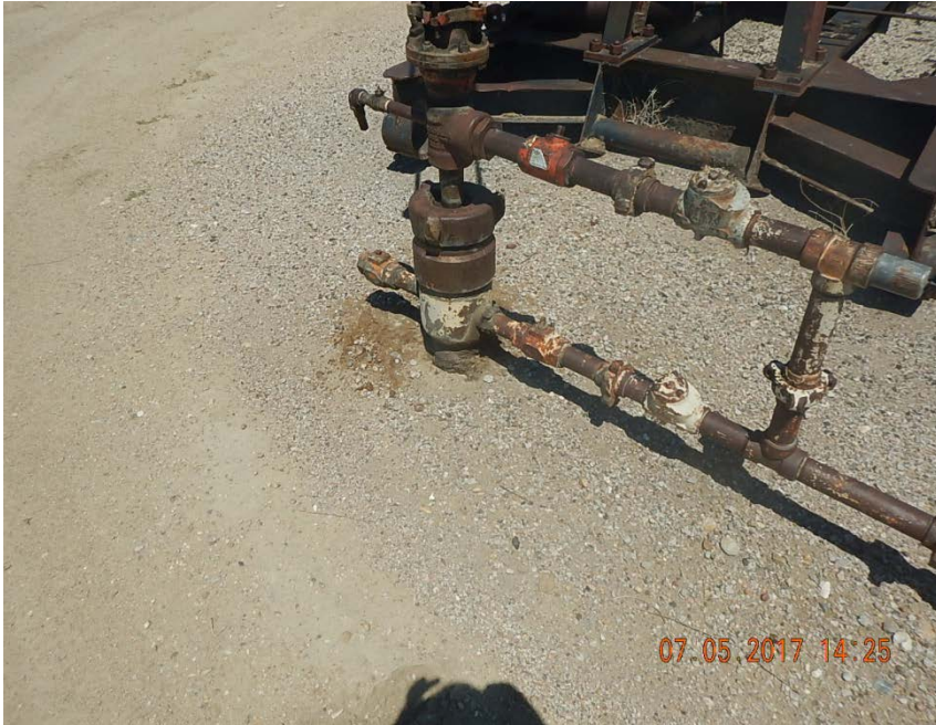
Photo 2: No bradenhead plumbed to surface
