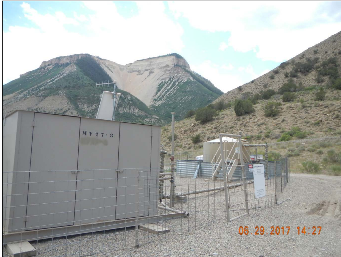
Separator and tank battery
