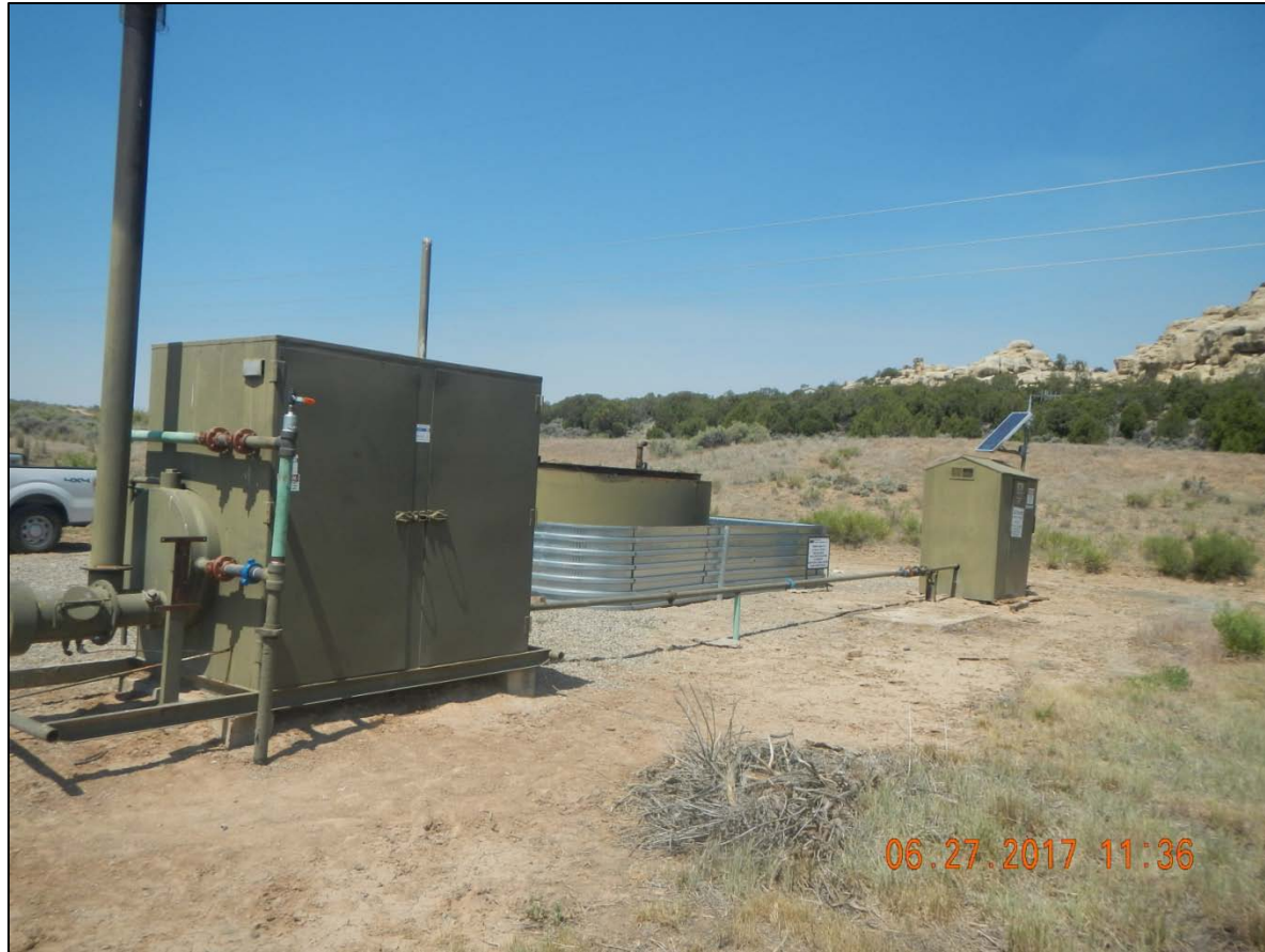
Separator , meter and, tank .
