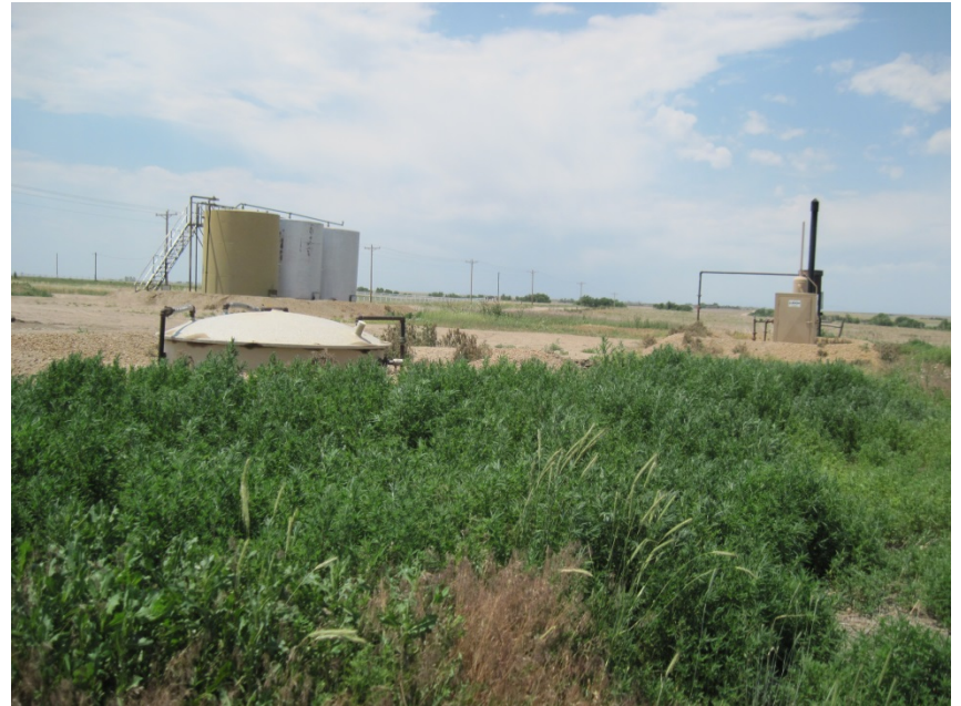
TANK BATTERY EQUIPMENT AND WEEDS
