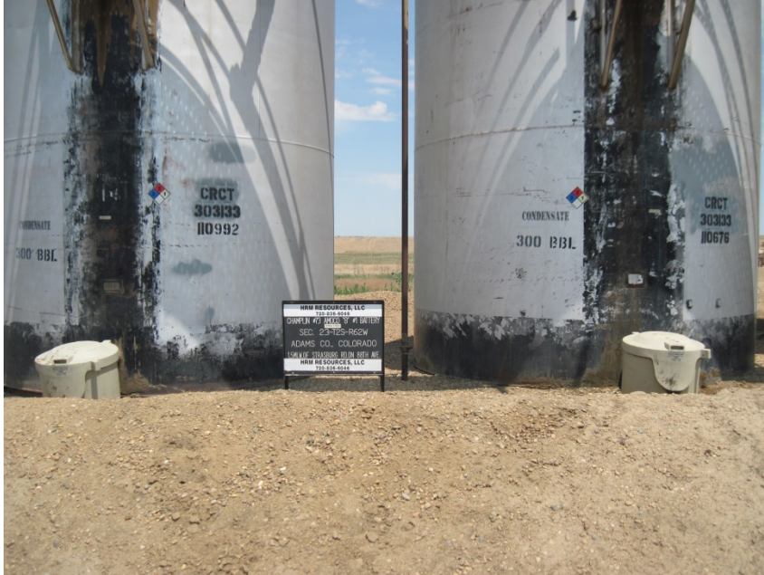
TANK BATTERY AND EQUIPMENT
