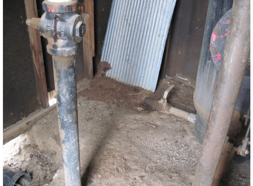
TREATOR HOUSE AND STAINED SOIL
