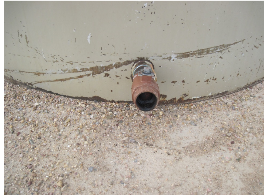
NO CAP ON PROD OIL TANK VALVE
