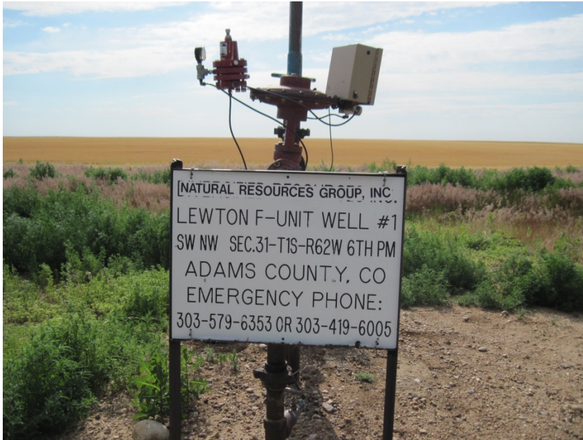
WELLHEAD LEWTON F UNIT #1 NO BRADENHEAD PLUMBED UP
