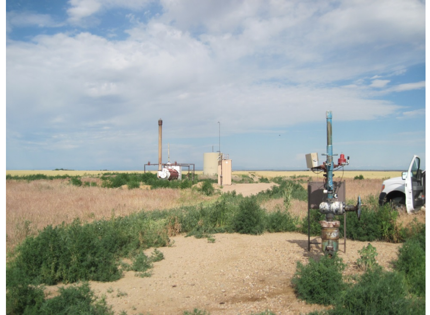
WELLHEAD AND LOCATION WEEDS
