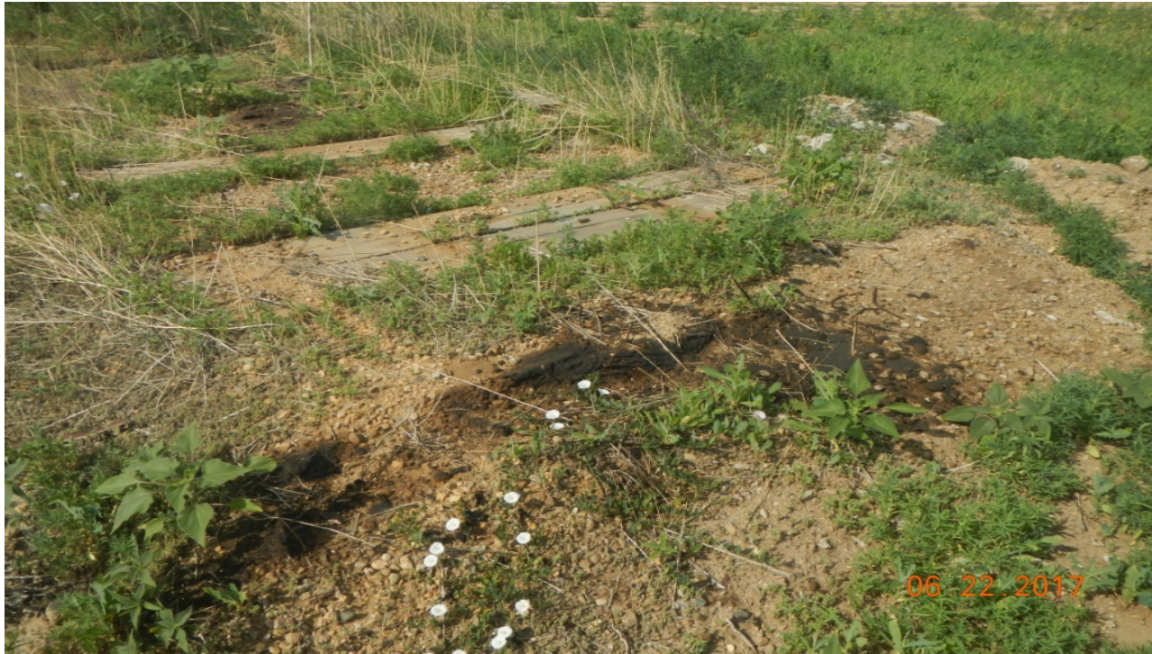
photo 5: There is wooden timbers and oil stained soil at the center of the location.
