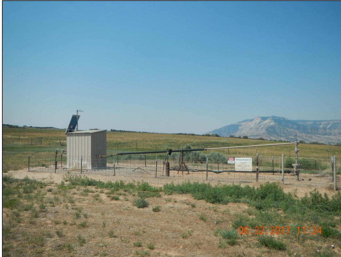
Well head, Meter and, Farm tap
