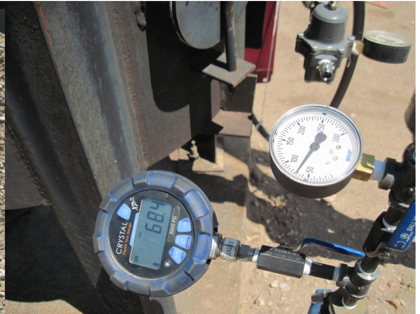
PRESSURE GAUGE AND RECORDER ECD 1" SUPPLY NGAS LINE
