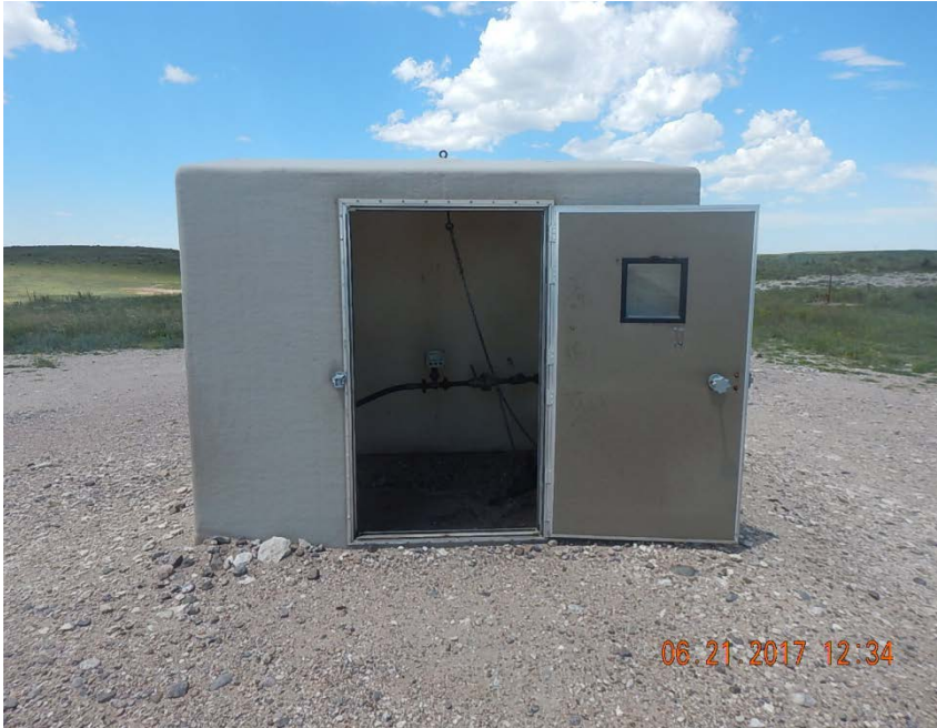
Photo 1: Wellhead, looking NW
