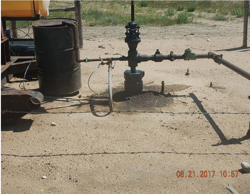
Photo 1: Stained soil at wellhead
