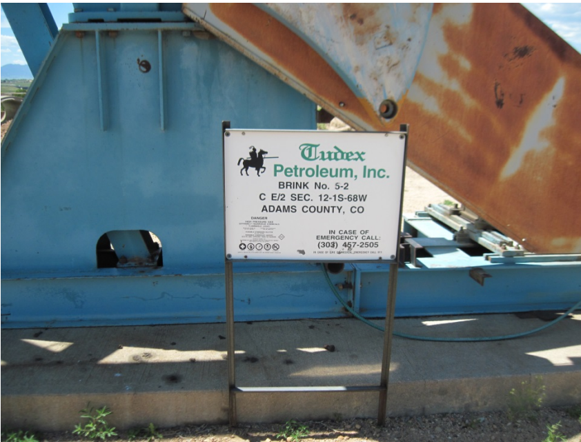
WELLHEAD SIGN, WRONG EMERGENCY NUMBER
