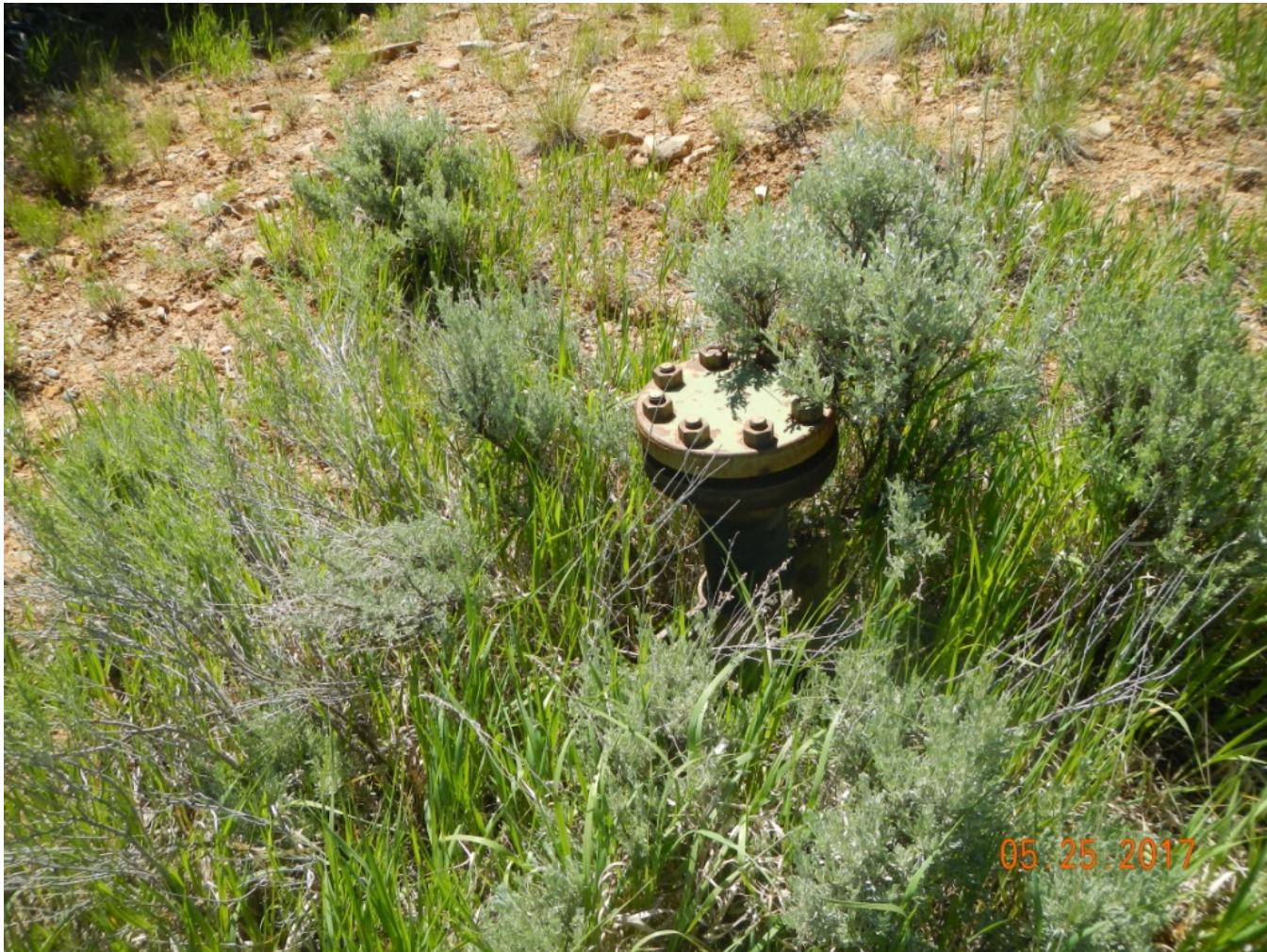
Photo 7. View of pipeline riser remaining within the project area at 37.11712 latitude and -108.14414 longitude.
