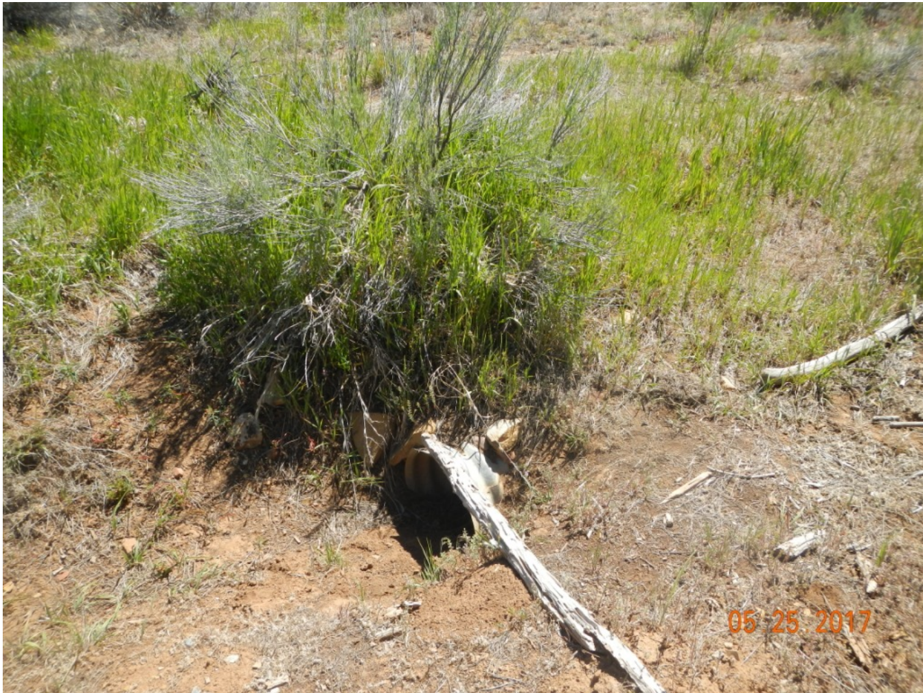
Photo 8. View of culvert still present along the access road near the entrance to the well pad.
