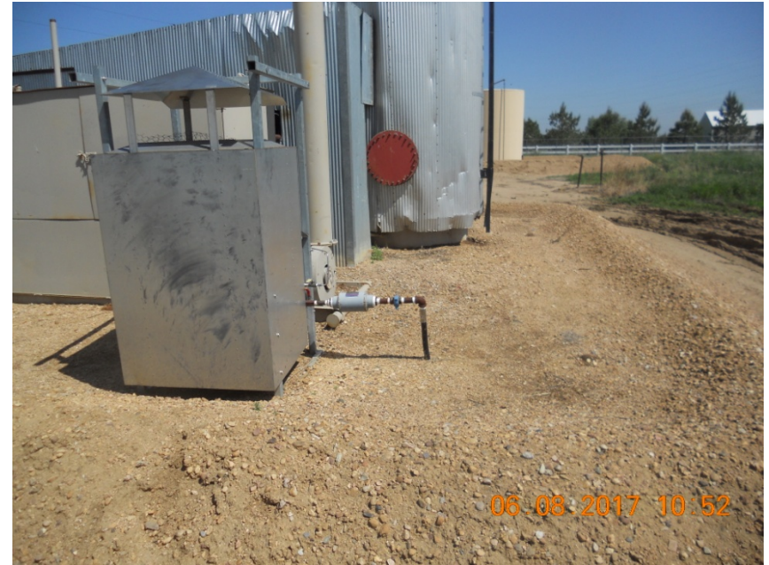
Photo 4. ECD and heater treater. Looking north
