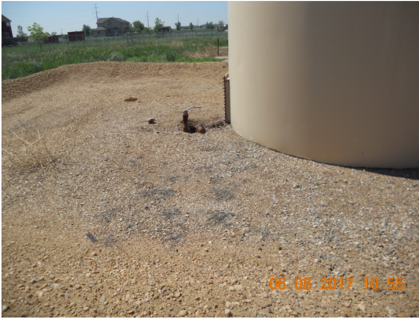
Photo 15. Looking south at eastside of production tank
