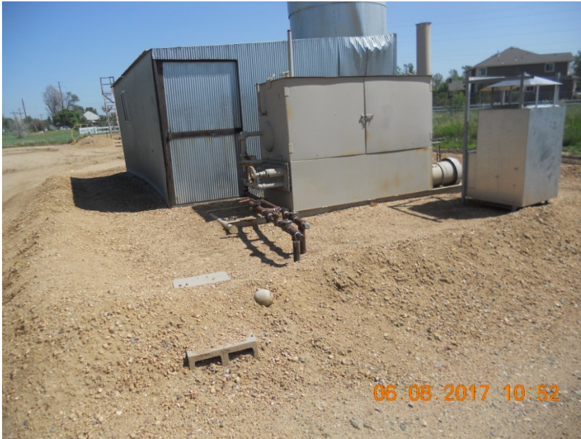
Photo 3. Separator, ECD. Looking north
