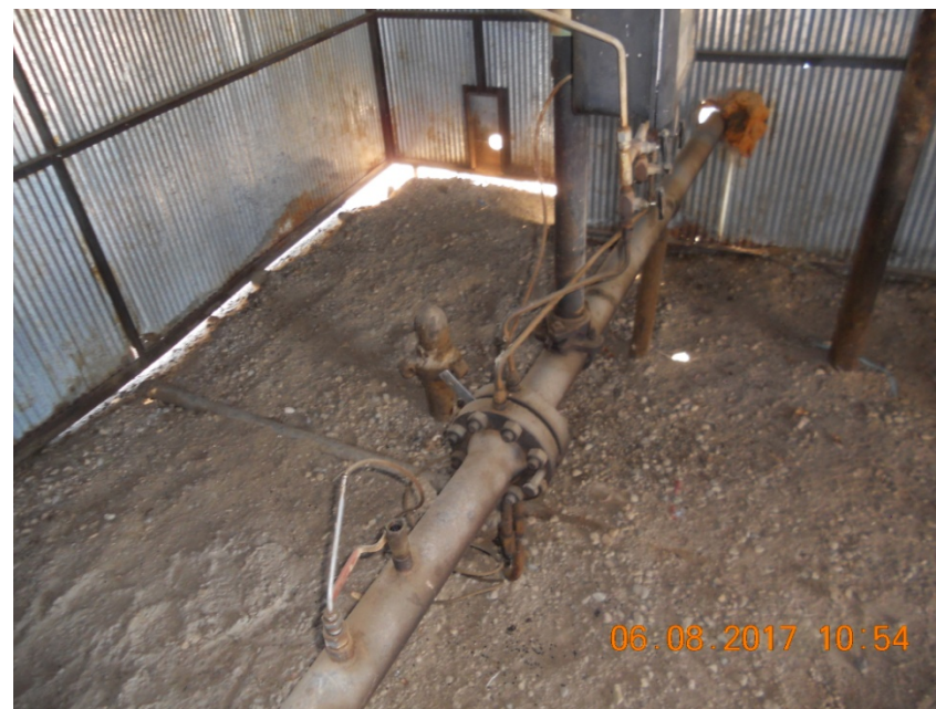
Photo 8. Unused 3-3" & 1-2" risers north of separator
