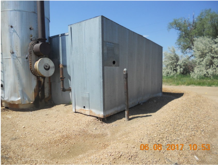
Photo 5. Riser north side of shed Not marked or tagged.
