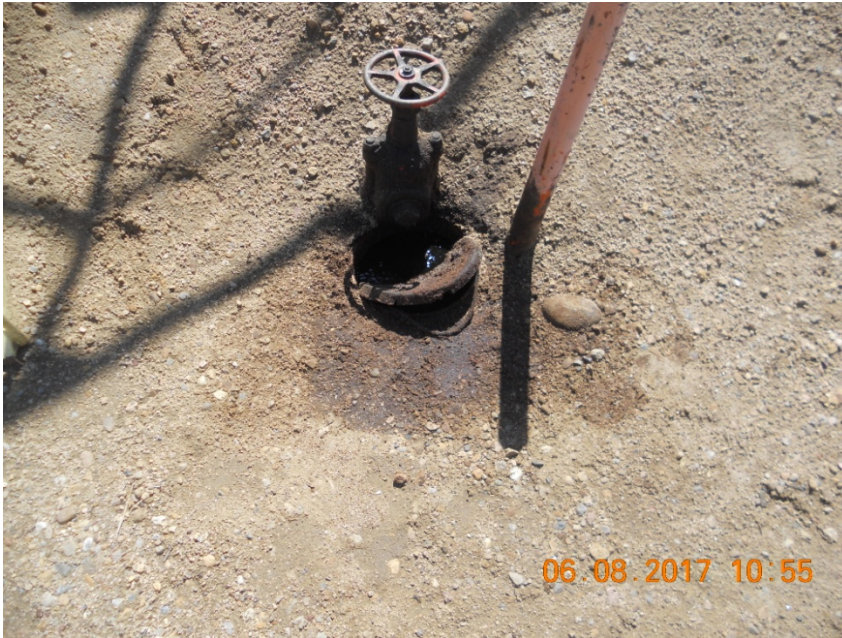
Photo 13. loadline spillage, No wildlife protection.
