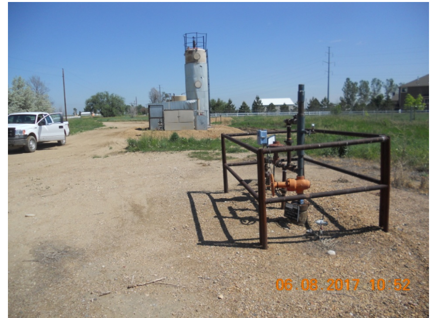
Photo 2. Wellhead and battery looking north
