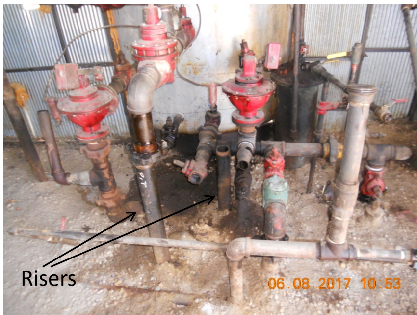
Photo 7. West side of heater treater. Note 2-3" line not hooked up
