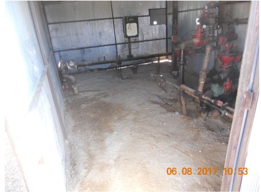
Photo 6. Inside treater shed. Note stained soil.
