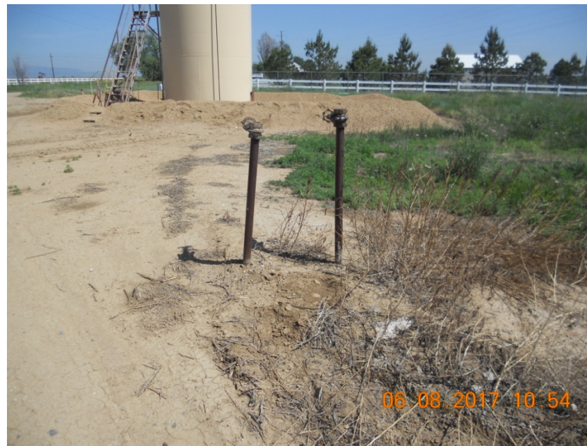
Photo 10. 2-2" riser between tank and separator/treater. Not marked or locked out
