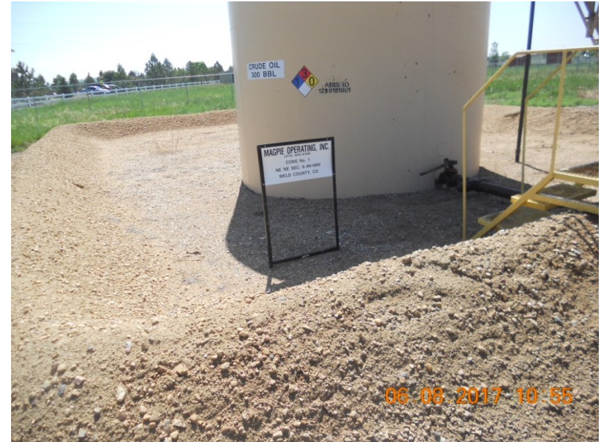
Photo 14. Sign at tank conflicts with location
