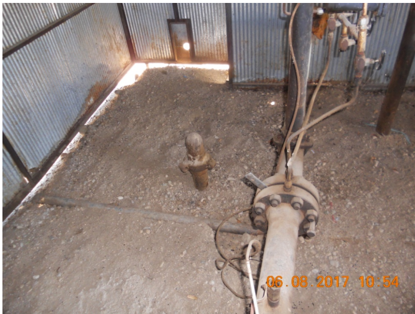
Photo 9. 3" riser in shed plugged not tagged or marked.
