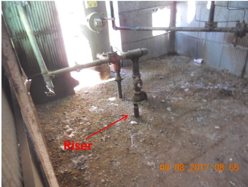
Photo 7. Used riser center of treater shed
