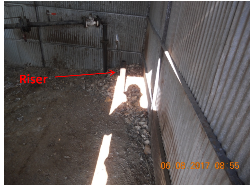
Photo 8. Unused riser NW corner treater shed
