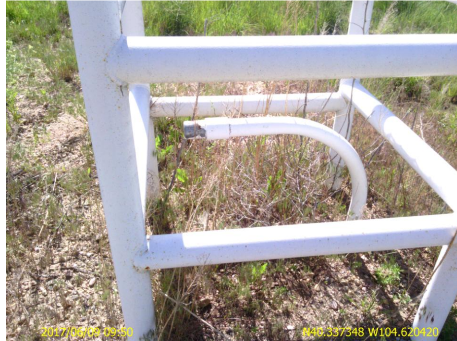
Photo 2: Photo taken from the tank battery location. Photo shows riser still remaining.
