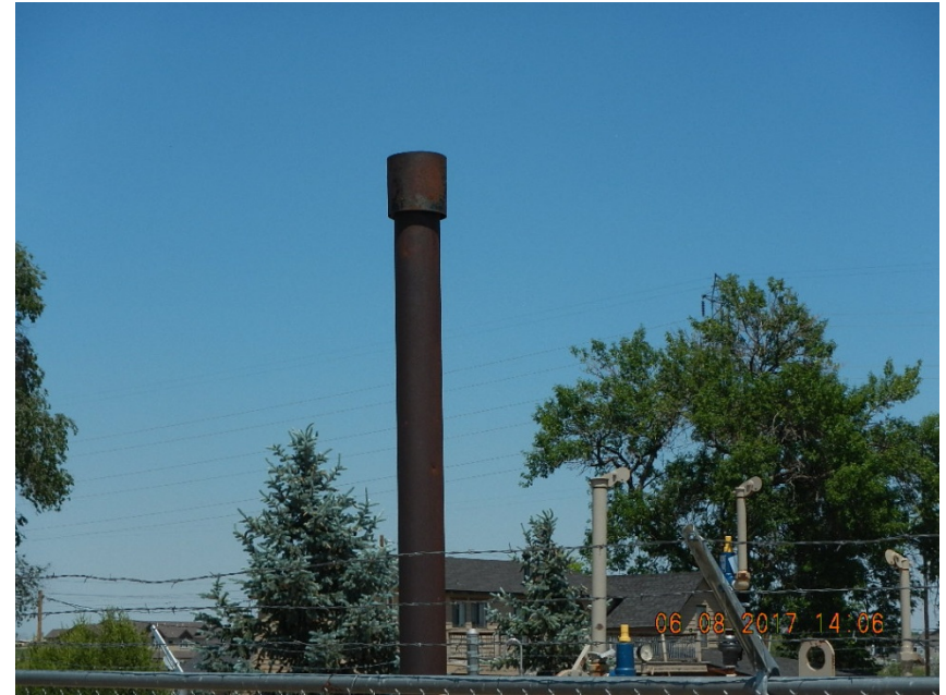
Separator burner stack
