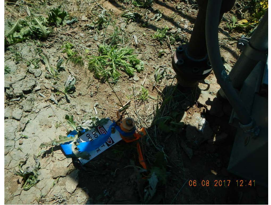
2" steel riser and 1" process riser
