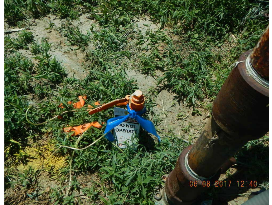
2" steel riser and 1" process riser
