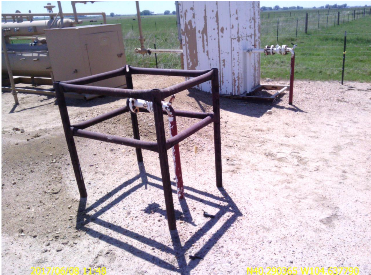
Photo 6: Photo taken from the tank battery south of the location. Photo shows riser located on the northwest corner of the horizontal separator. Riser does not have the required markings, or lockout/tagout required per the May 2, 2017 Flowline or Pipeline NTO. Riser will need to be removed per Phase II of the NTO.
